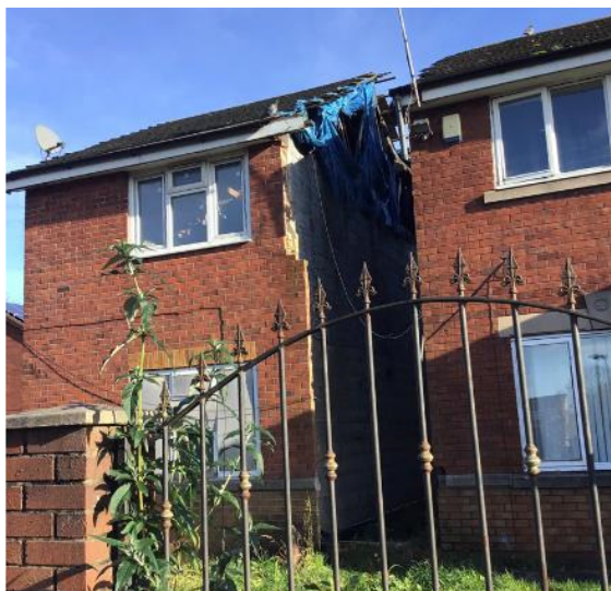
South aspect of demolished building with large open void. Pigeon recorded nesting.
