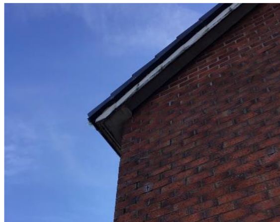
North aspect of building. Gaps between the wooden soffits and brick work. Present on north-east and north west corners.
