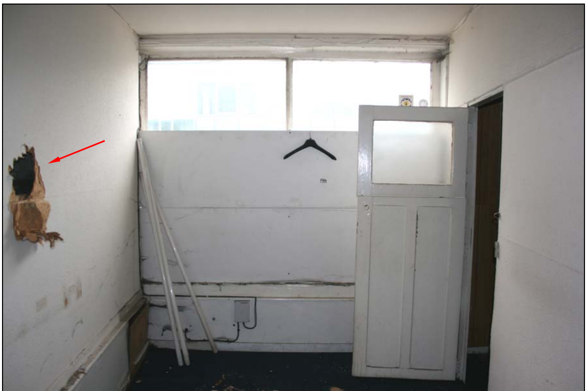
20. Looking to front of main room with probably mid-20 th century door to reception; void behind boarded wall indicates chimneybreast within
