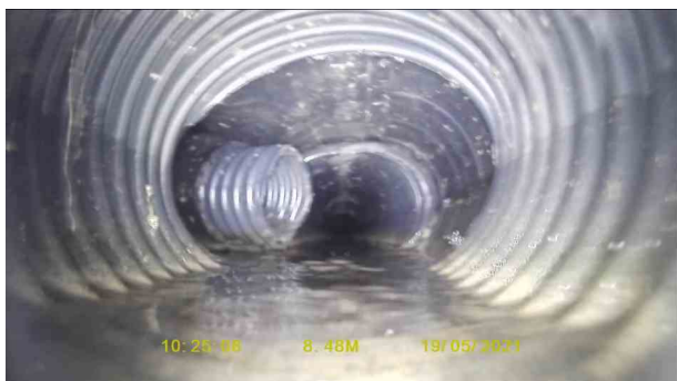
3, 00:00:58, 8.48 m Deformed sewer or drain, 10%
