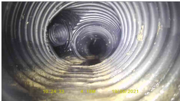
1, 00:00:22, 4.06 m Deformed sewer or drain, 5%
