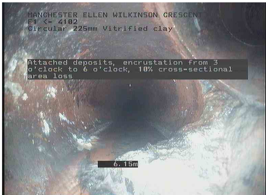
F1X_88f46f24-c831-48b2-8274-98e42e457bbe_20210528_094946_561.jpg, 00:01:39, 6.15 m Attached deposits, encrustation from 3 o'clock to 6 o'clock, 10% cross-sectional area loss
