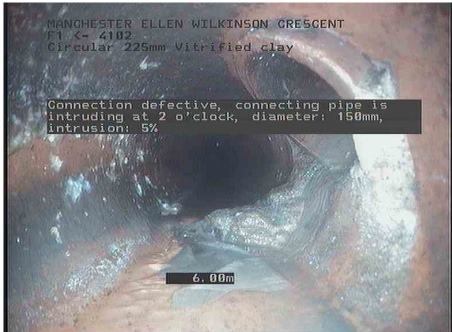
F1X_c6ccb4a9-1e3b-463f-b38b-864e26e7da76_20210528_094927_694.jpg, 00:01:28, 6.00 m Connection defective, connecting pipe is intruding at 2 o'clock, diameter: 150mm, intrusion: 5%
