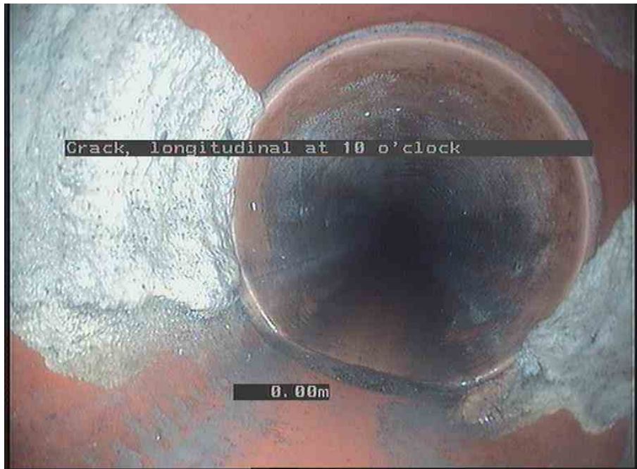
F1X_d86d64c4-f1a9-4ede-8dd2-538740c4dd34_20210528_094751_541.jpg, 00:00:08, 0.00 m Crack, longitudinal at 10 o'clock
