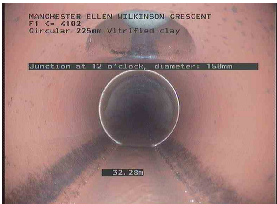
F1X_6ed753d6-9658-445c-ae76-81d1c2599358_20210528_095332_887.jpg, 00:05:05, 32.28 m Junction at 12 o'clock, diameter: 150mm, APPEARS TO BE CAPPED OFF
