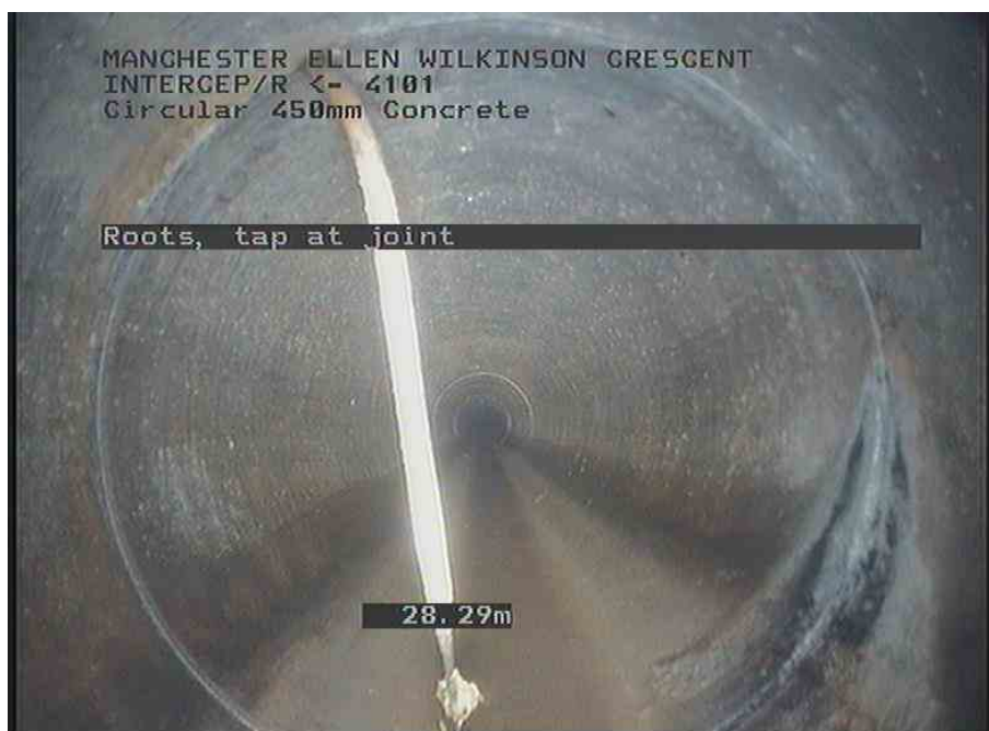
INTERCEP_RX_c812ce8b-762b-461e-a7ab-e9543cf060c3_20210528_084754_115.jpg, 00:02:53, 28.29 m Roots, tap at joint
