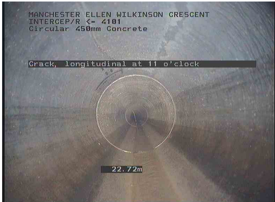
INTERCEP_RX_bf316faa-fd0a-474b-b224-6eec861e4035_20210528_084719_303.jpg, 00:02:21, 22.72 m Crack, longitudinal at 11 o'clock
