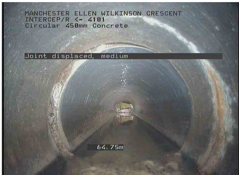
INTERCEP_RX_1b64a4a2-ccde-4c70-92da-dc94153e0c3c_20210528_085145_416.jpg, 00:06:02, 64.75 m Joint displaced, medium
