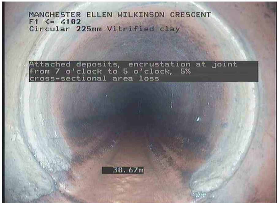
F1X_e9be66f6-579a-4379-b30a-0f6c88459fbe_20210528_095439_621.jpg, 00:06:02, 38.67 m Attached deposits, encrustation at joint from 7 o'clock to 5 o'clock, 5% cross-sectional area loss
