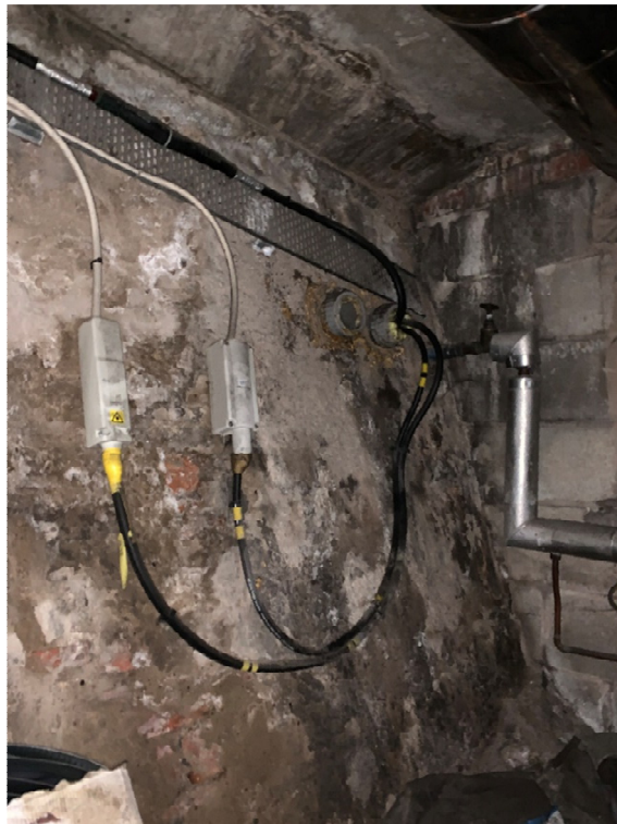
Existing incoming BT ducts (with one spare)
