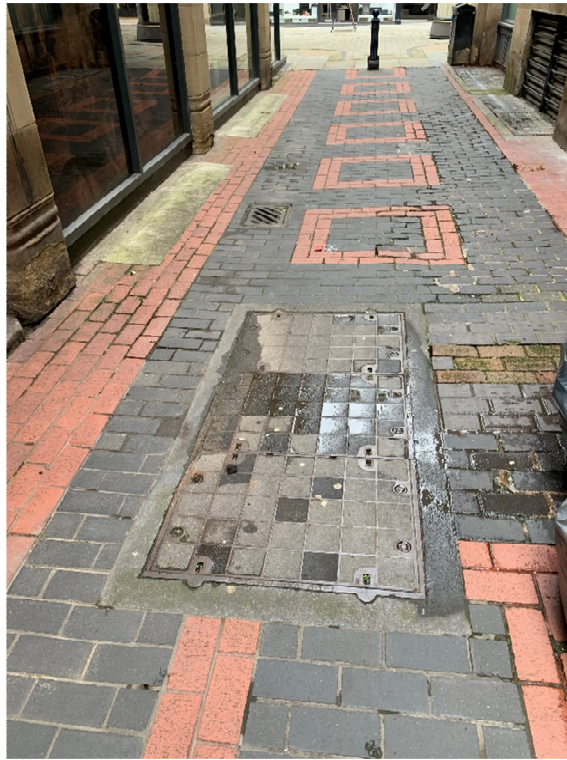
Existing cable chambers in Four Yards
