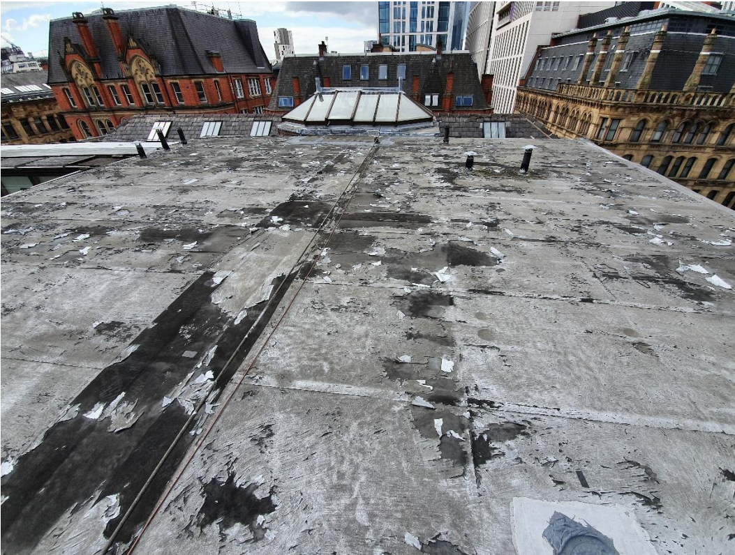
3. General condition of the flat roof covering, peeling and evidence of localised patch repairs.
