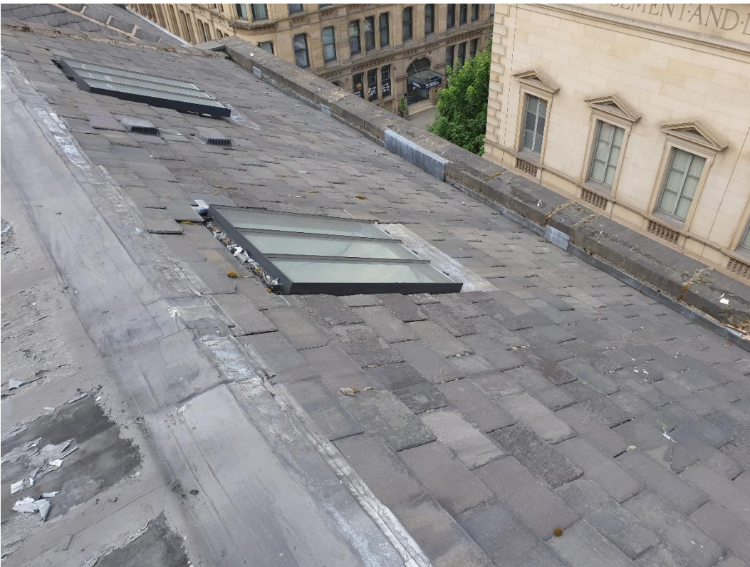
4. Poor detailing of the junction between the flat roof and the slate covered mansard. Note lead patch repairs to gutter.
