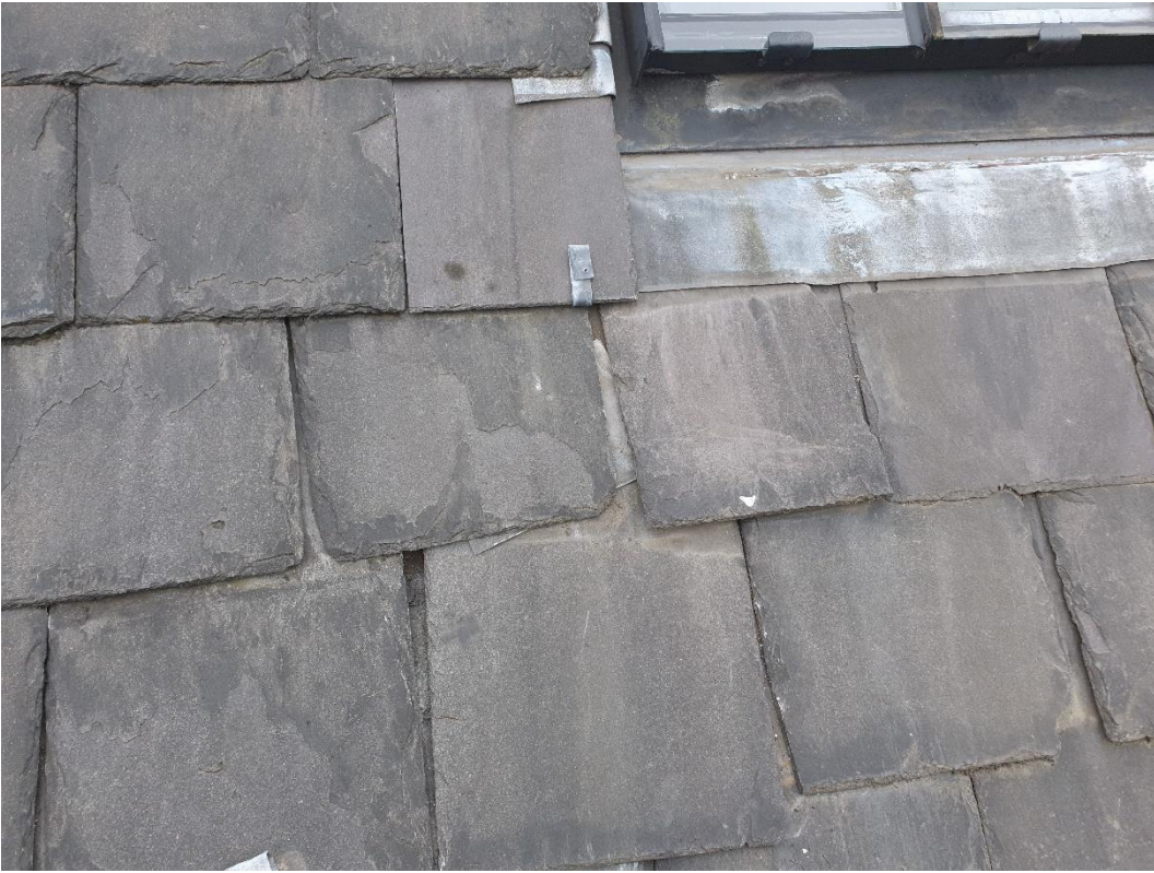
13. Uneven and poorly repaired slates.
