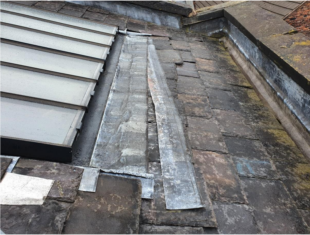
17. Displaced lead flashing beneath rooflight window.
