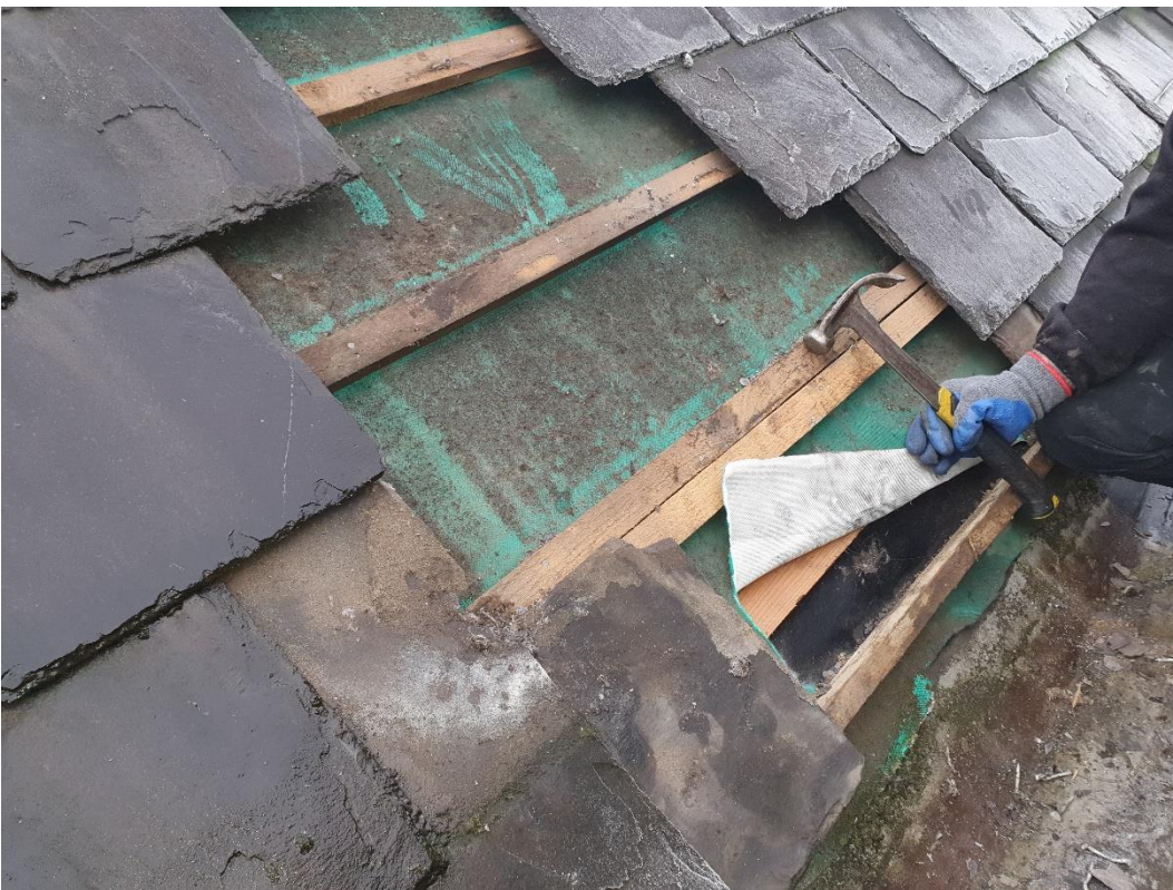
20. Investigation of pitched roof, showing “tight” roof felt and untreated timber battens.
