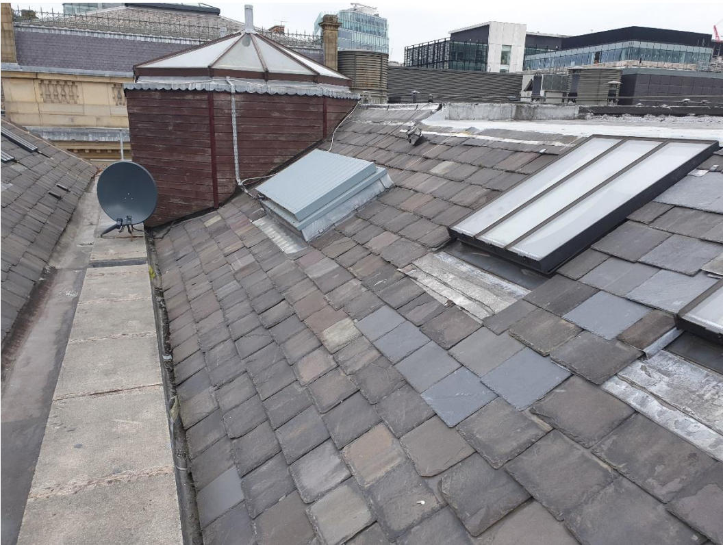
14. Poorly matched and fitted slate repairs.
