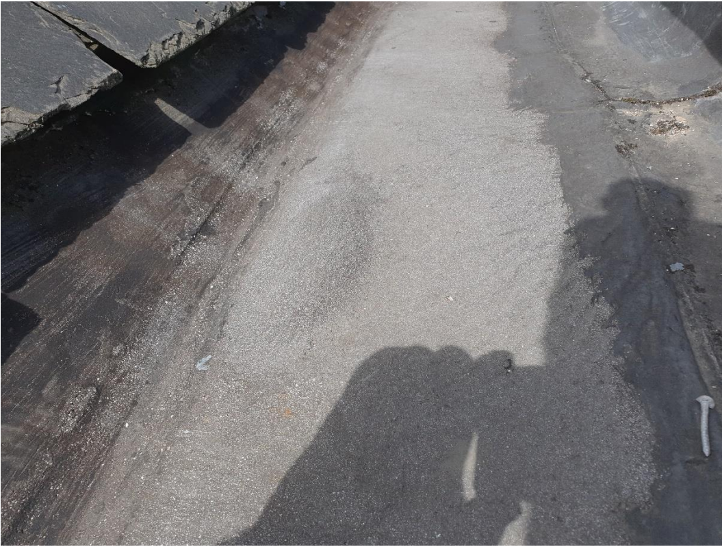
11. Blistering to bitumen coated valley gutter.
