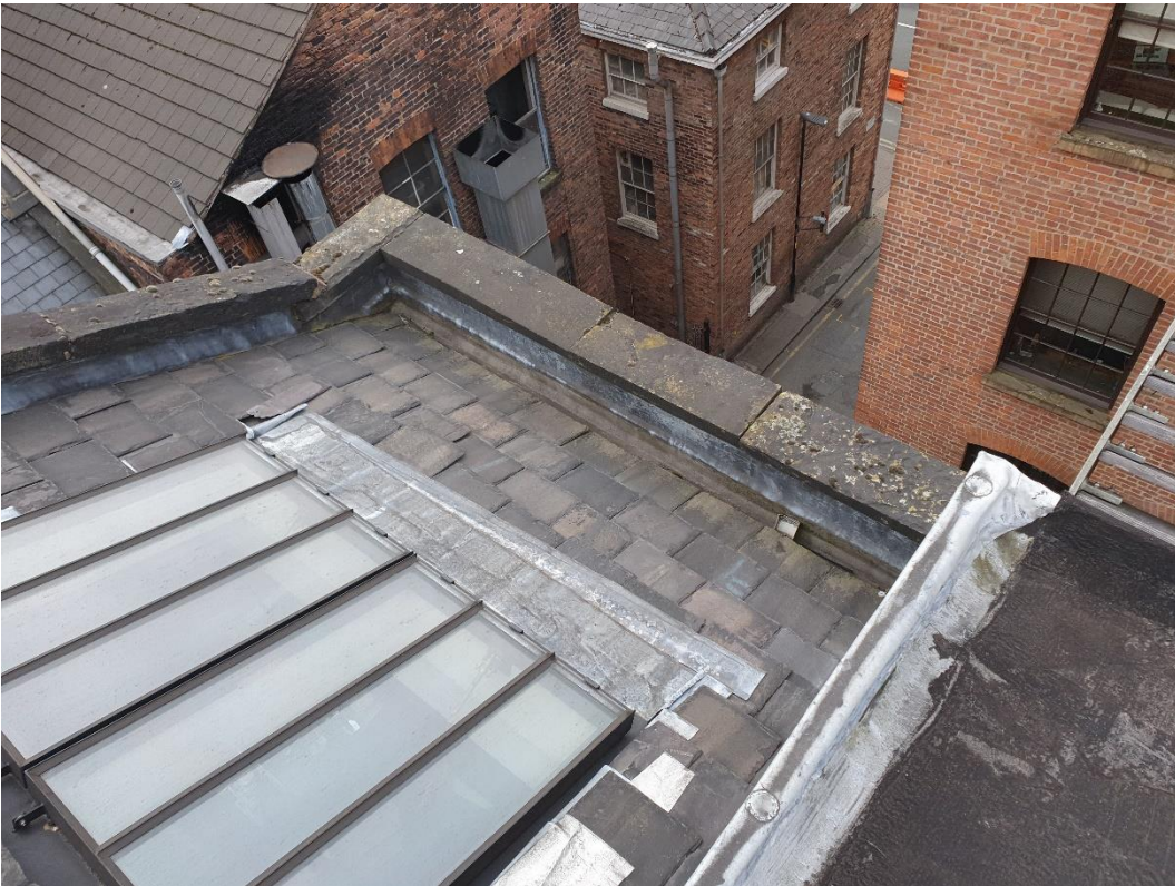
12. Poor condition of mortar joints to stone copings.
