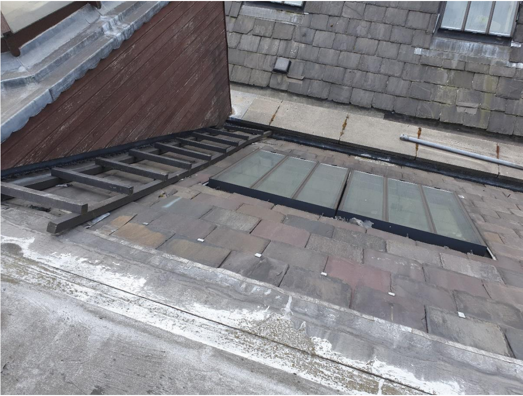
5. Timber access ladder to valley. Timber cladding to stairwell atrium is heavily aging.
