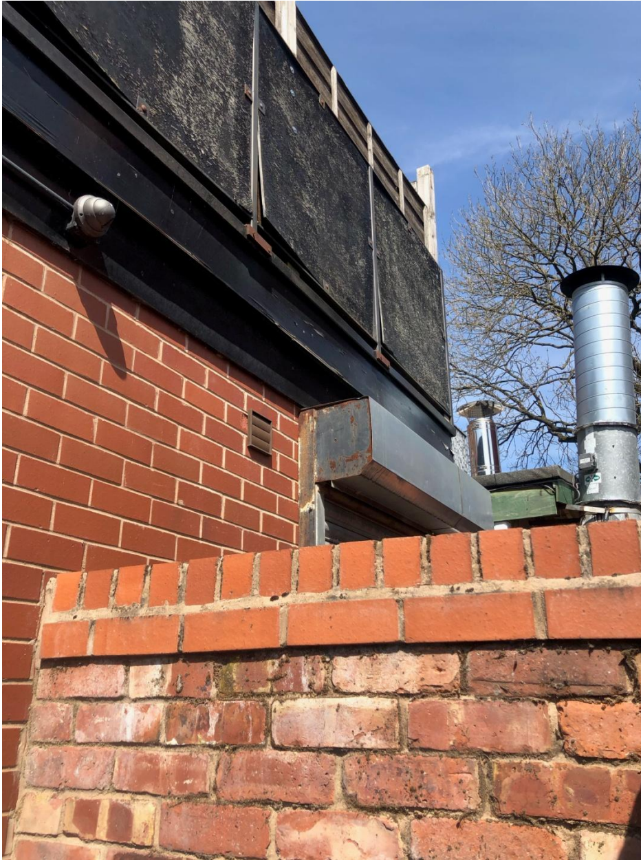
Above: Neighbouring extract flues showing discharge below eaves with downward deflecting hat cowlings
