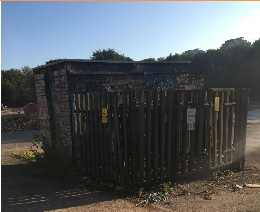
PLATE 5: VIEW OF EXISTING ELECTRICAL SUBSTATION
