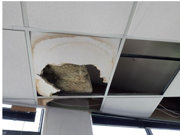
Plate 4.20: Broken Suspended Ceiling Tile with Insulation Cages Above.
