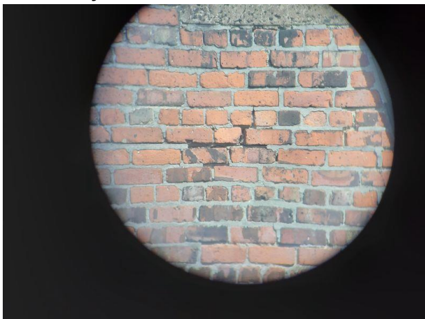
Plate 4.3: Minor Missing Mortar which did not Extend.
