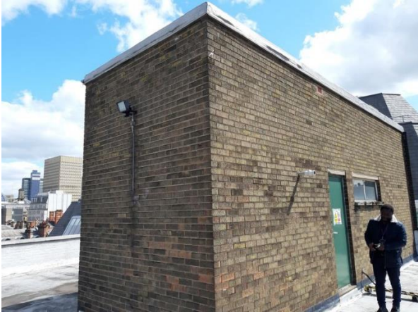
Plate 4.17: Motor Room on Roof of Grange House.
