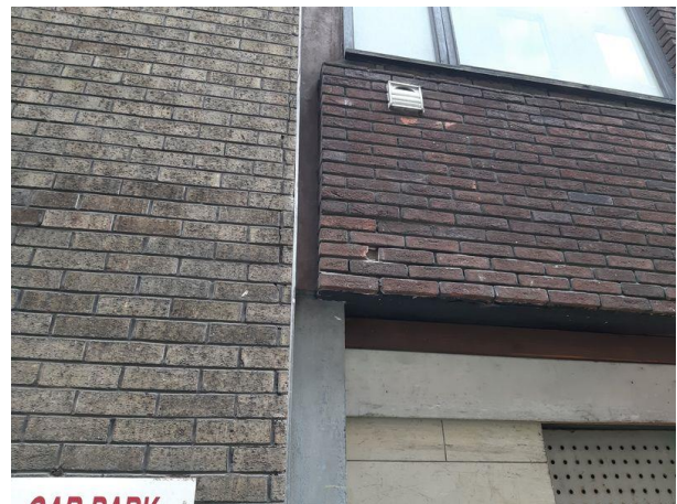
Plate 4.11: Broken Brick-style Panel to the East with Concrete Behind.
