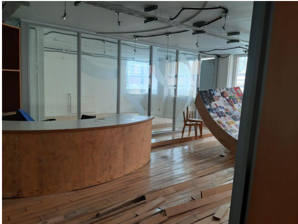
Plate 4.14: Dance Studio on First Floor with Degraded Flooring.
