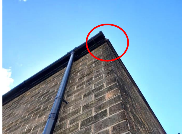
Plate 4.18: Small Cobwebbed Gap Below North-west Section of Fascia Board.
