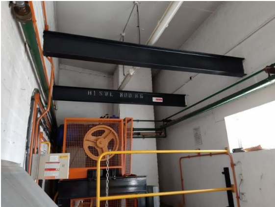
Plate 4.21: Lift Motor Room on Roof of Grange House.
