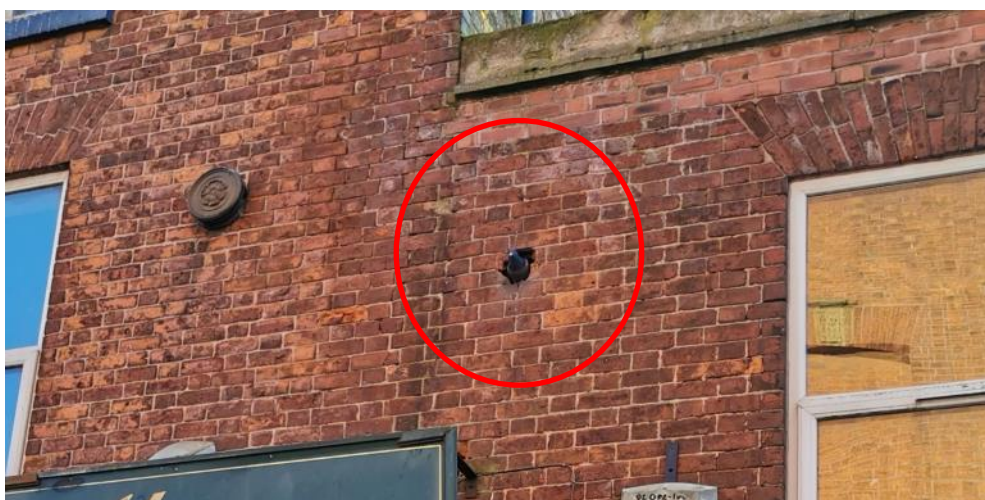
Plate 4 - Note the presence of Feral Pigeon ( Columba domestica 'livia') exiting the building via damage in the brickwork
