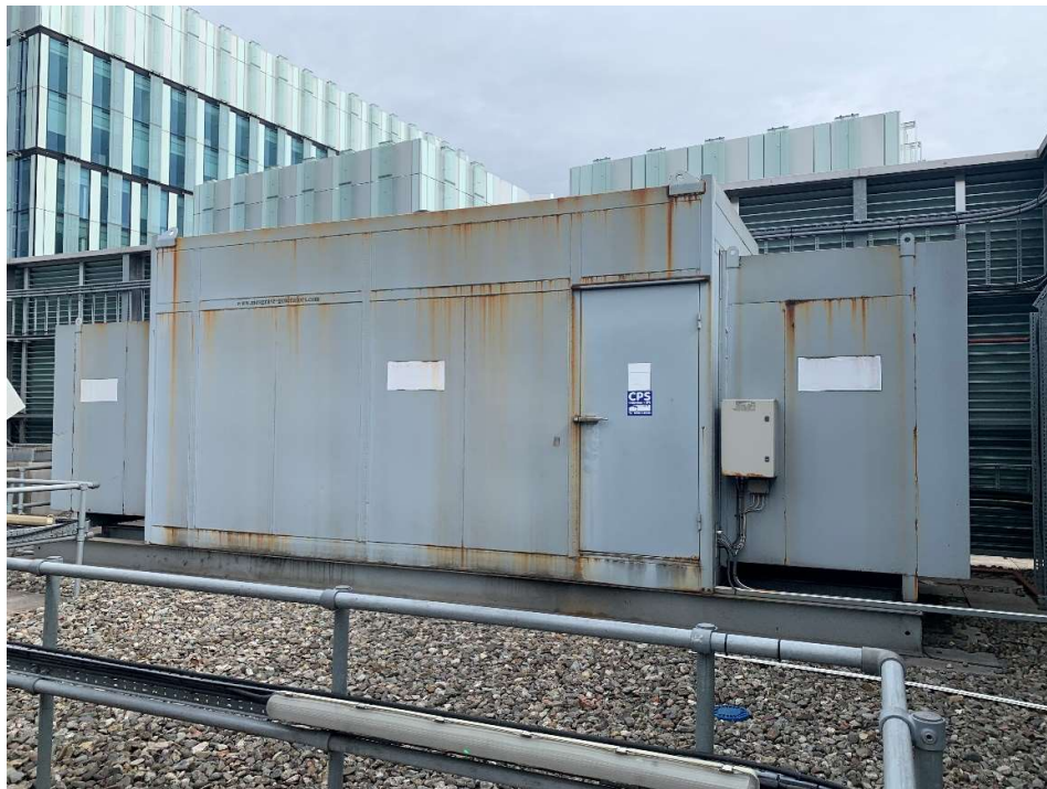
Rooftop Plant Area – Existing Plant Equipment (Generator)
