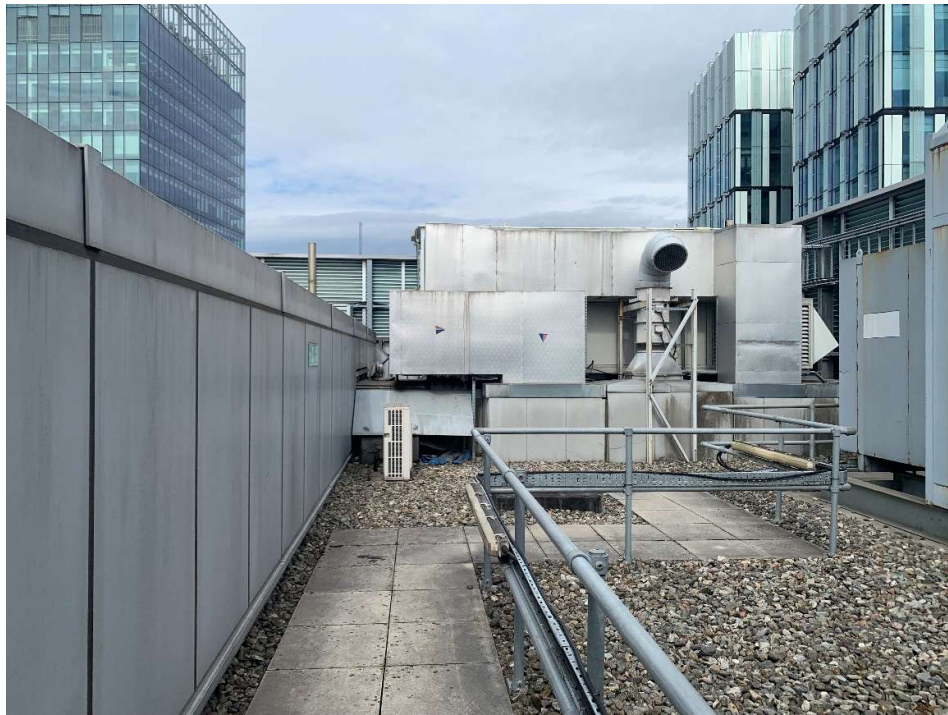
Rooftop Plant Area – Existing Plant Equipment (Air Handling Units)
