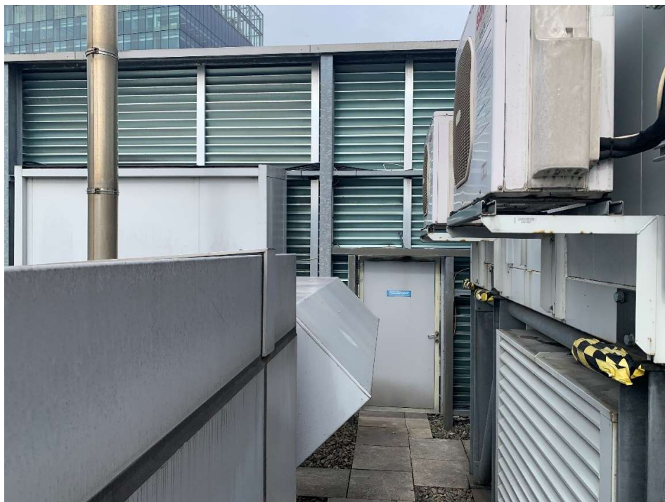
Rooftop Plant Area – Existing Plant Equipment (Extract and A/C Condensers)
