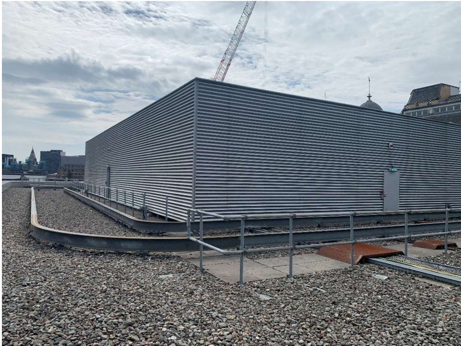
Rooftop Plant Shield
