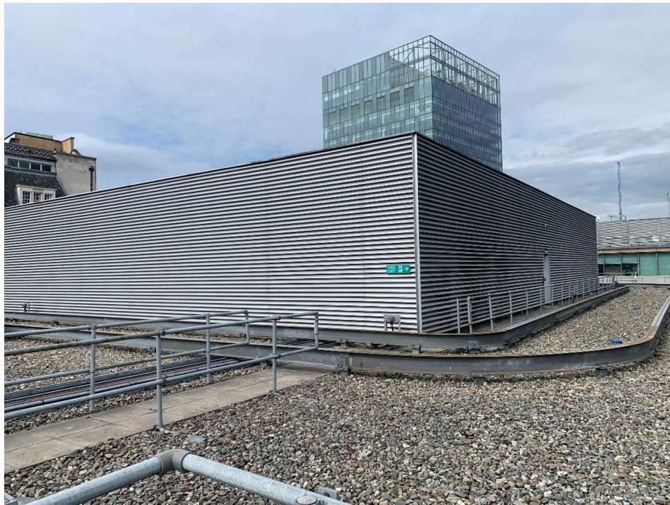
Rooftop Plant Shield
