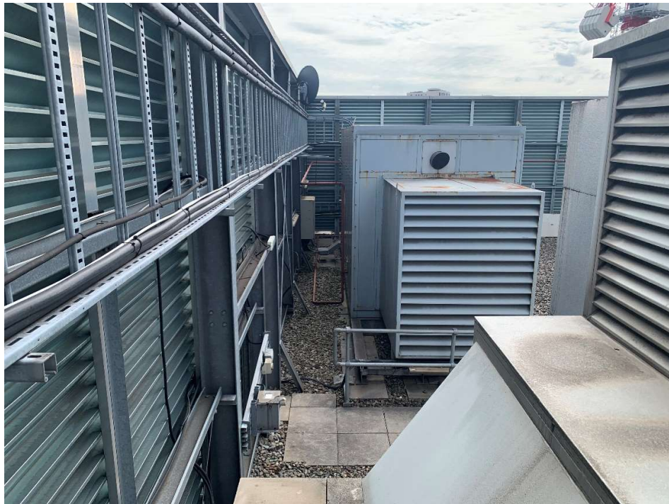
Rooftop Plant Area – Existing Plant Equipment (Generator)
