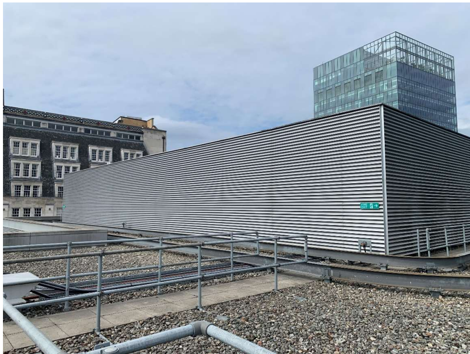
Rooftop Plant Shield
