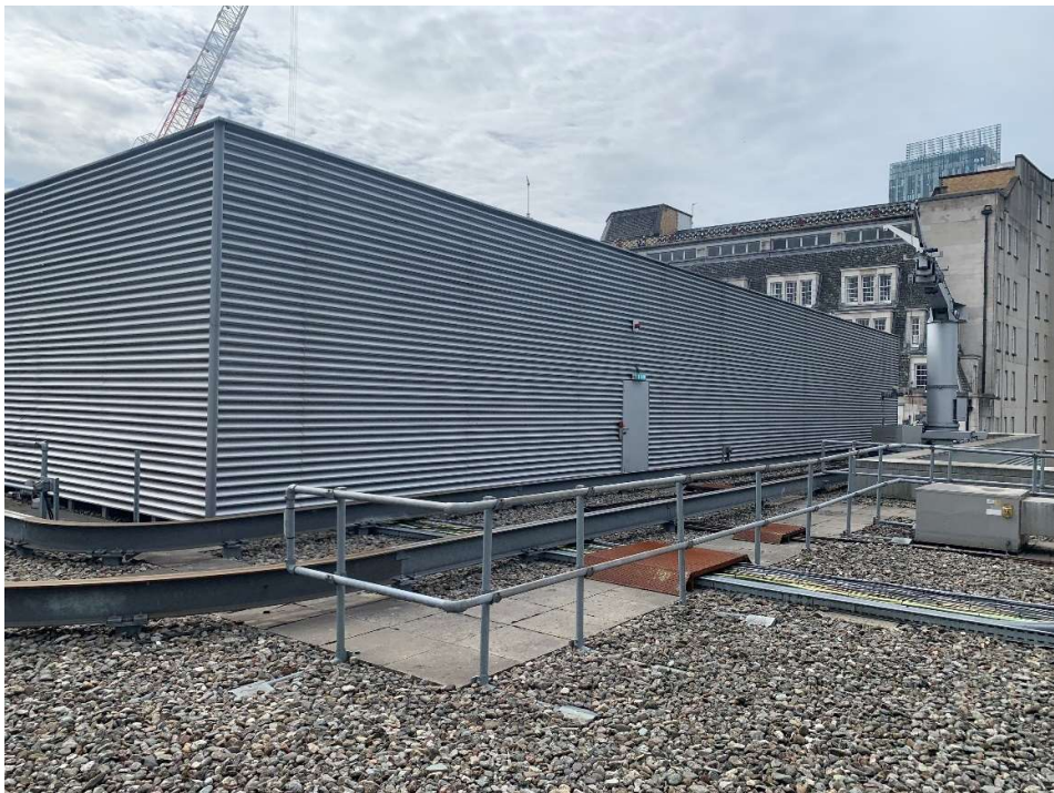
Rooftop Plant Shield
