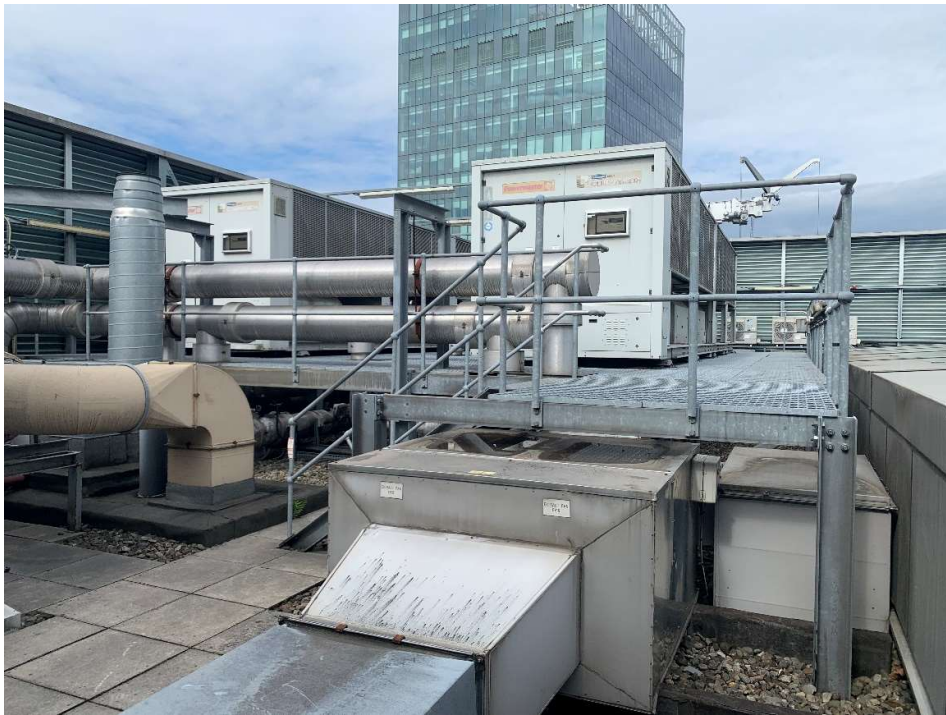
Rooftop Plant Area – Existing Plant Equipment (Chillers)
