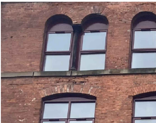
2. Damaged pointing above window head and widow cill to window above. Repointing required with mortar to match existing.
