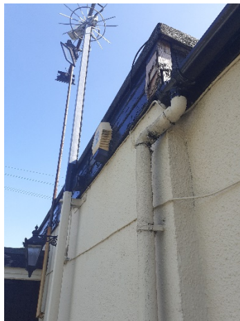
Figure 20: Small gap in the roof panels/barge boards under the eaves of the overhang at the rear/western wall of the main building B1. Low potential.
