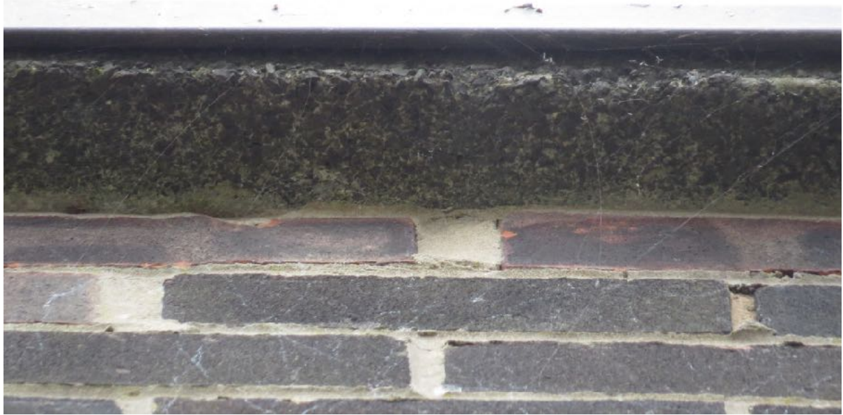
3 – Concrete capping stones on the end walls are tightly fixed with no suitable gaps.
