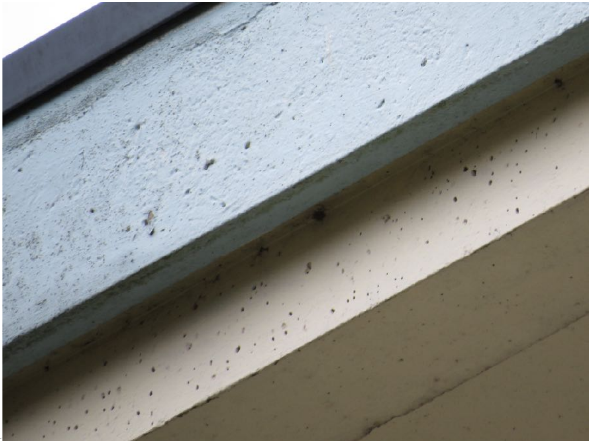
4 – There are no fascia boards, and no gaps between roofing materials and walls.
