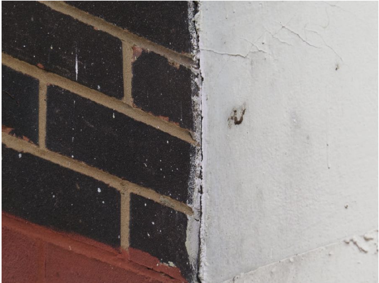
5 – There are no gaps between rendered walls and brickwork.
