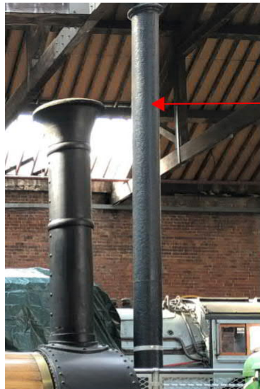
Hollow column acting as rainwater pipe
