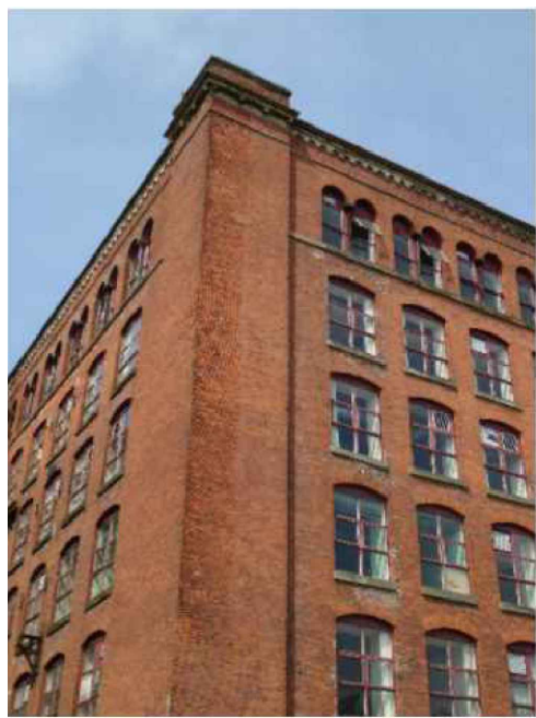
3. Check condition of existing mortar on southern corner, full height of building. Repoint where necessary with mortar to match existing.
