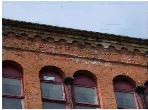
1. Water ingress causing salt to appear on face of brick. Water ingress to be resolved, brickwork to be cleaned.
