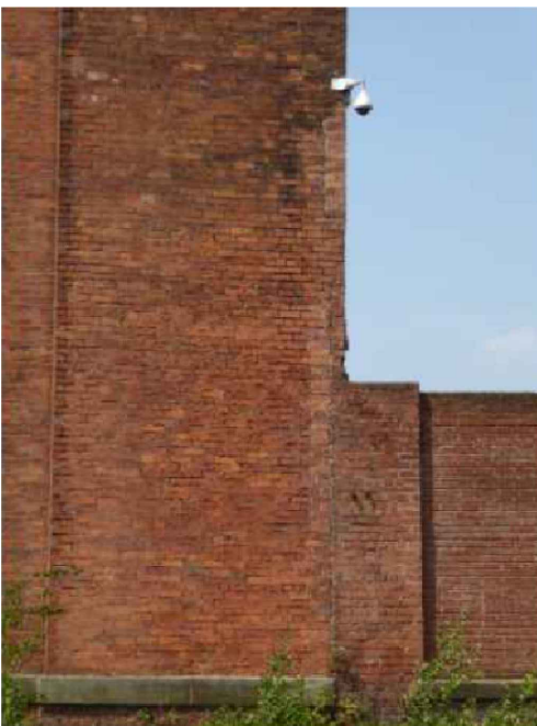
5. Poor pointing of brickwork. Rake out existing mortar and repoint with mortar to match existing.
