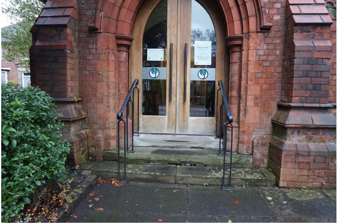
Figure 5 : Existing Entrance (South Porch) to Church. There is no accessible path for the users with disabilities.
