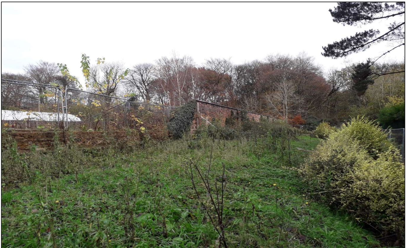
Photo No.6 – View along South Elevation Boundary Wall to Horticultural Centre – Section of wall has collapsed completely.
