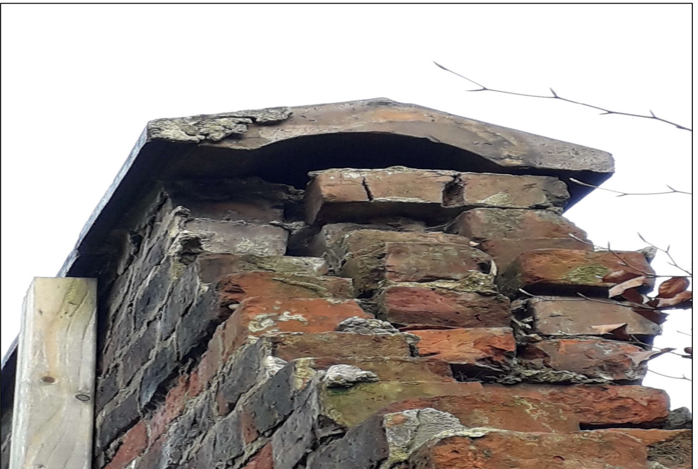
Photo No.4 – View showing cross section of boundary wall where collapse has occurred.
