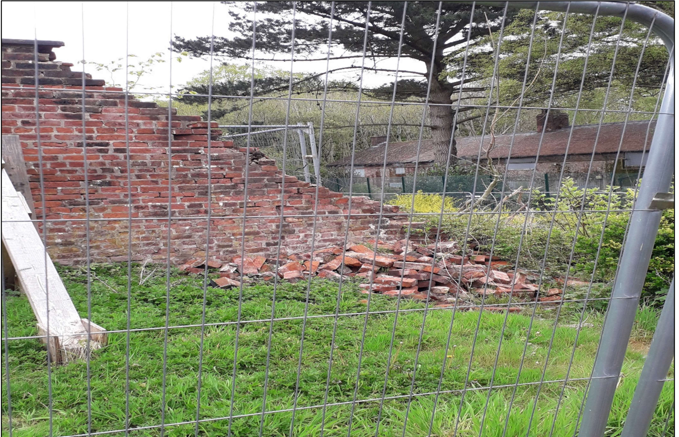
Photo No.3 – View of collapsed section of the West Elevation Boundary Wall where it meets the Southern Boundary to the Horticultural Centre.
