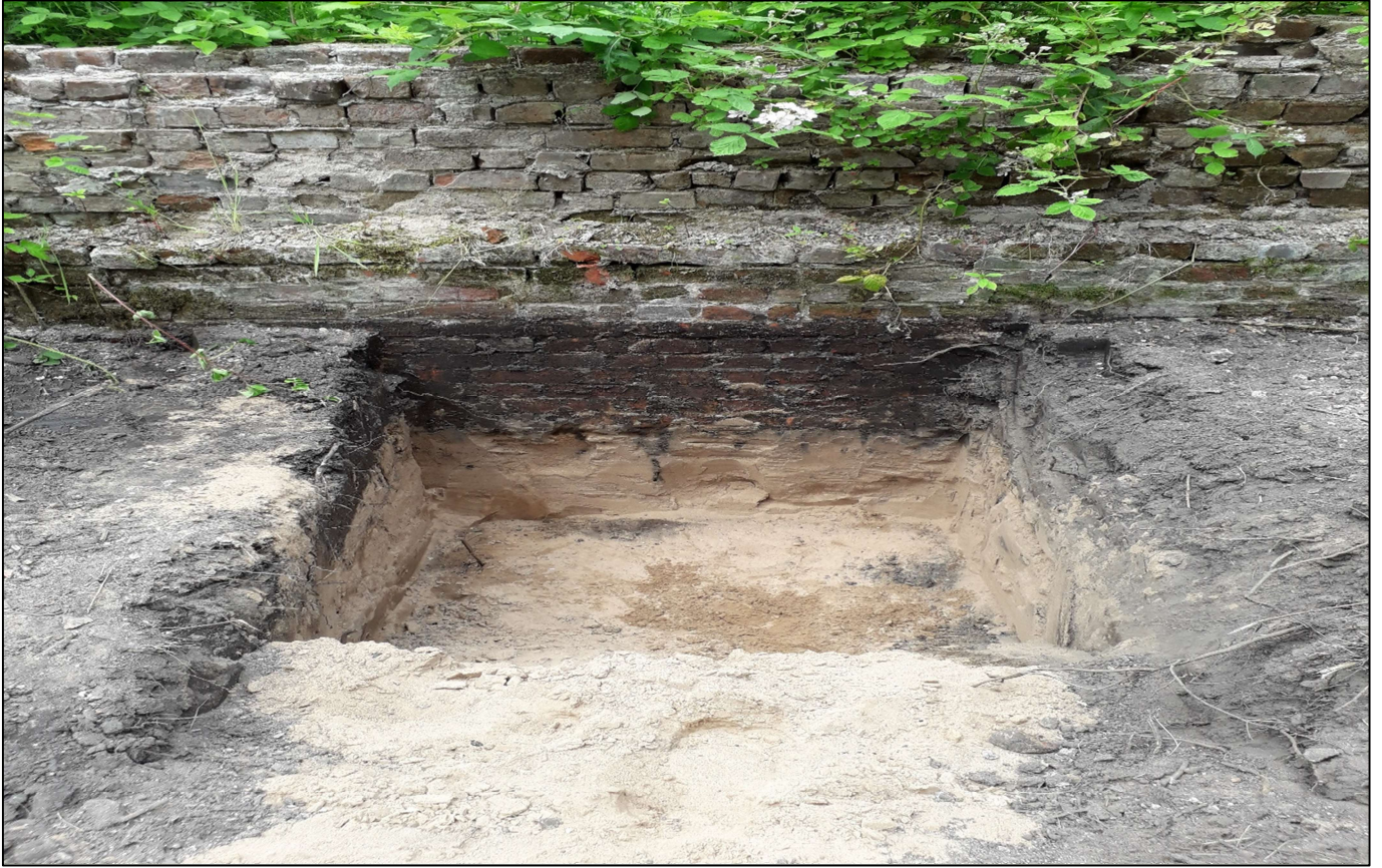
Photo No.7 – View of trail hole at base of collapsed section of South Elevation Boundary Wall to Horticultural Centre. Wall was originally built with no foundation in sandy sub-strata.
