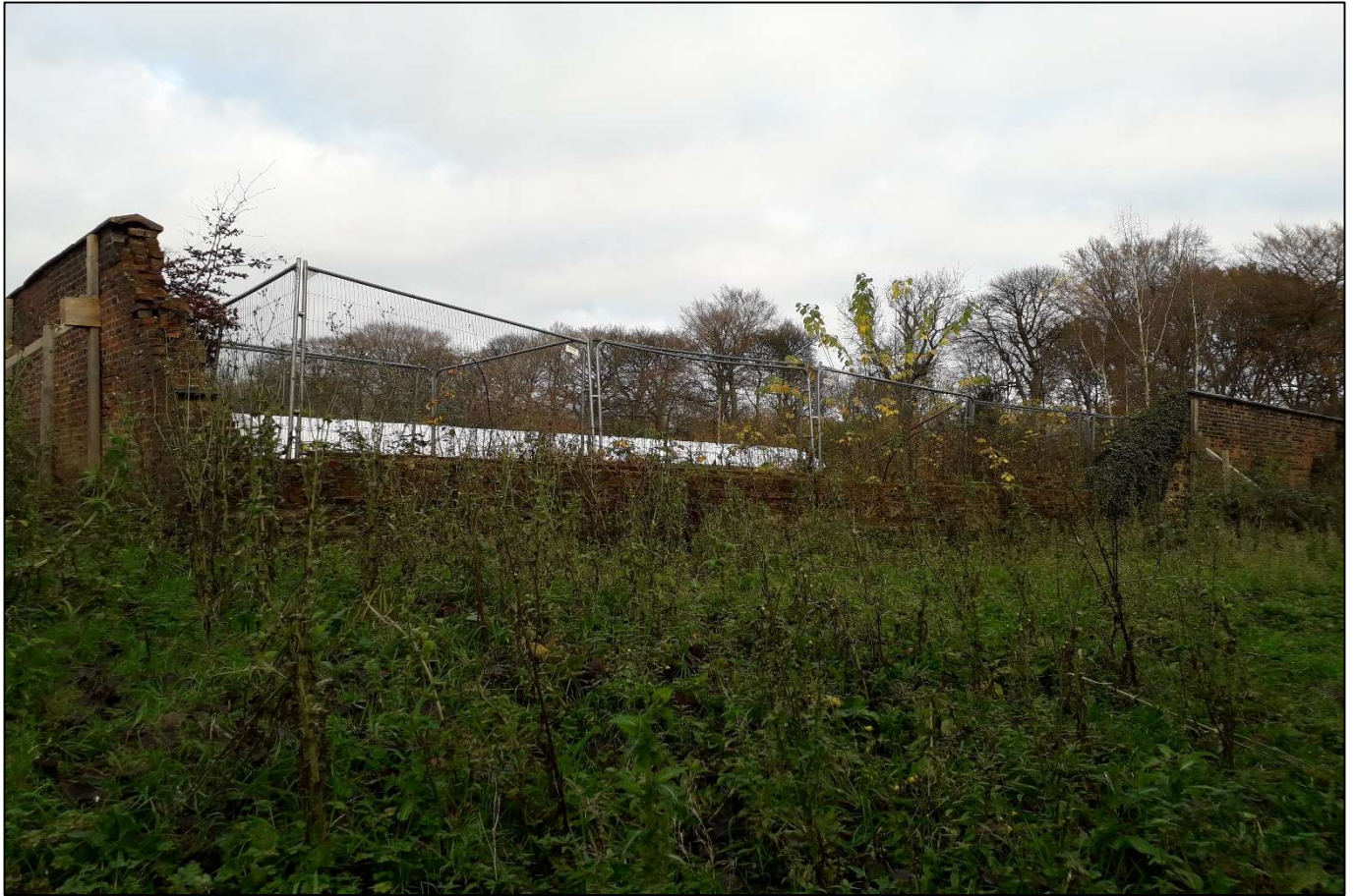
Photo No.5 – View along South Elevation Boundary Wall to Horticultural Centre – Section of wall has collapsed completely.
