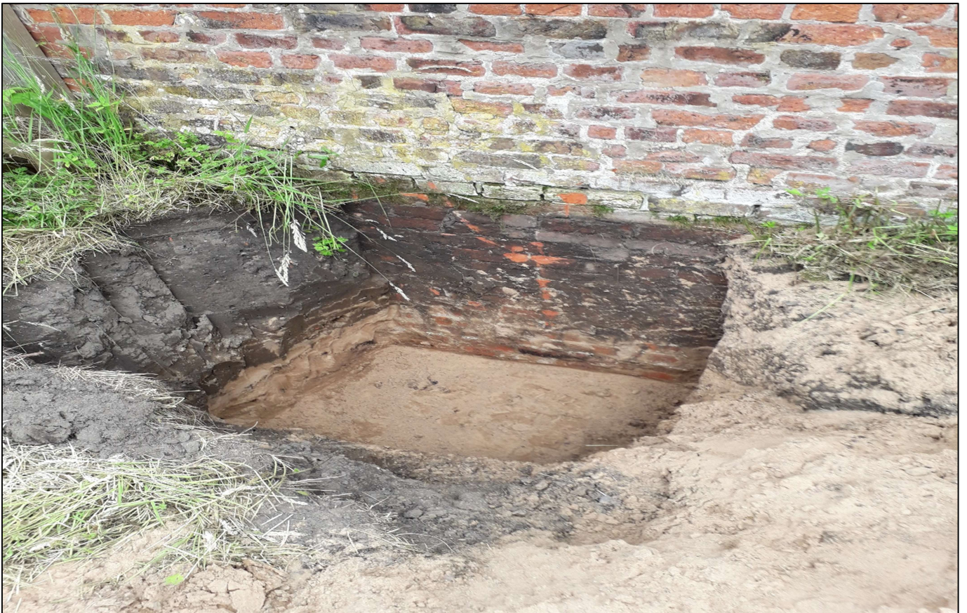
Photo No.8 – View of trail hole at base of West Elevation Boundary Wall to Horticultural Centre. Wall was originally built with no foundation in sandy sub-strata.
