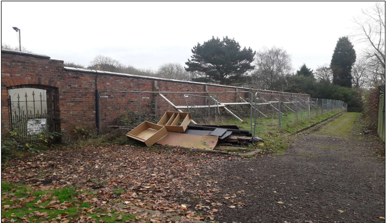
Photo No.1 – View along the West Elevation Boundary Wall to the Horticultural Centre. Due to the walls instability, the area adjacent to it has been cordoned off and temporary raking shores erected.
