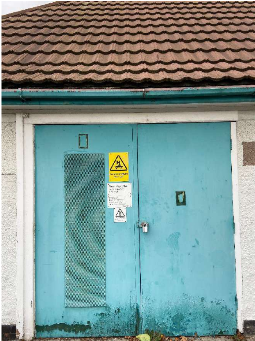
Photograph 2 – Electricity substation located in the west of the site, adjacent to the sites entrance
