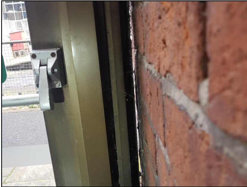
Photograph 2 showing the gap in one of the floor to ceiling windows
