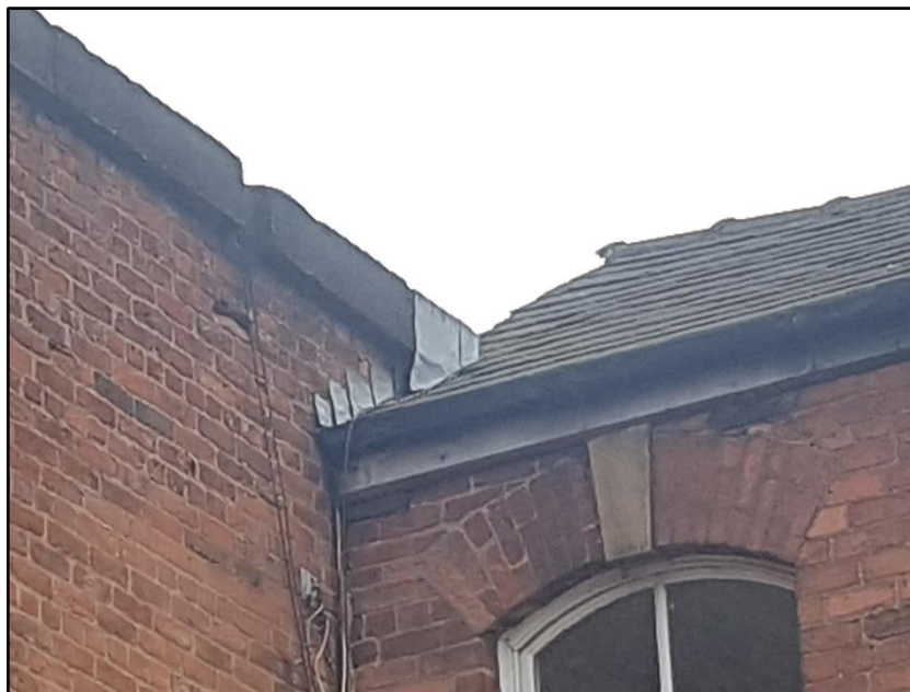
Photograph 5 showing the loose flashing at the western elevation
