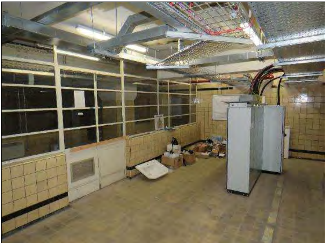
Figure 1a: The former bank switch gear room now used for hotel services. The glazed screen is an original feature.
