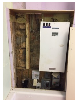
Wall mounted services
