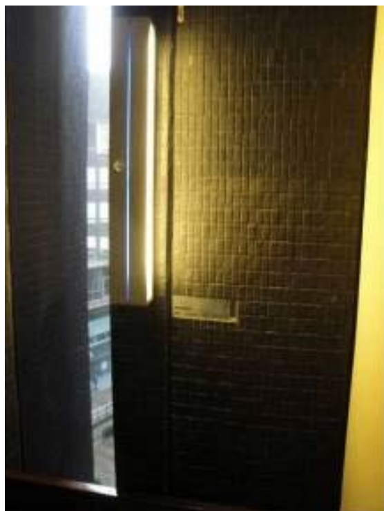
Figure 32: The original concealed smoke vent when closed, note the poor level of lighting. (Photo taken in 2017; condition has since deteriorated)
