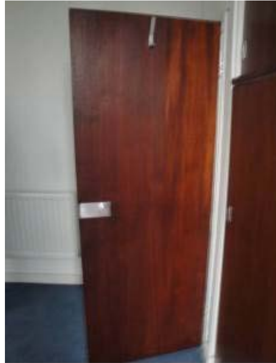
Figure 49: An example of the original doors (not solid) with simple chrome handles. (Photo taken in 2017; condition has since deteriorated)
