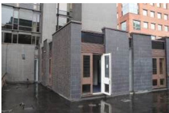
Figure 50: Looking north-west towards the caretakers flat from the roof terrace, showing the four pairs of original timber French doors. (Photo taken in 2017; condition has since deteriorated)
