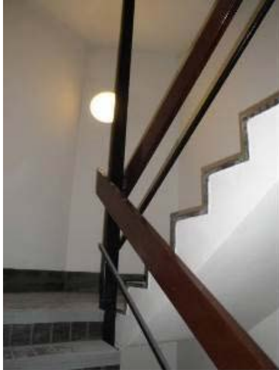
Figure 30: The King Street Block fire escape, showing the original al balustrade and blue brick flooring. (Photo taken in 2017; condition has since deteriorated)
