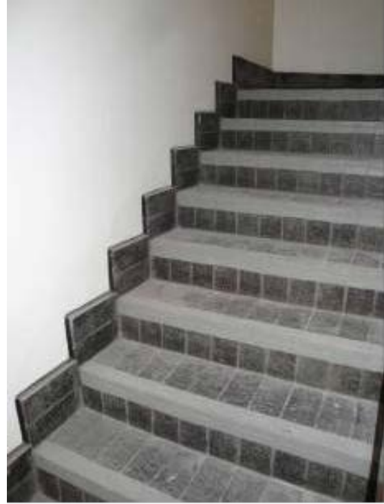
Figure 31: The King Street Block fire escape showing the original blue brick flooring and skirting. (Photo taken in 2017; condition has since deteriorated)
