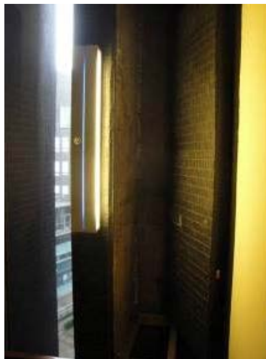
Figure 33: The smoke vent as it appears when pushed open. (Photo taken in 2017; condition has since deteriorated)
