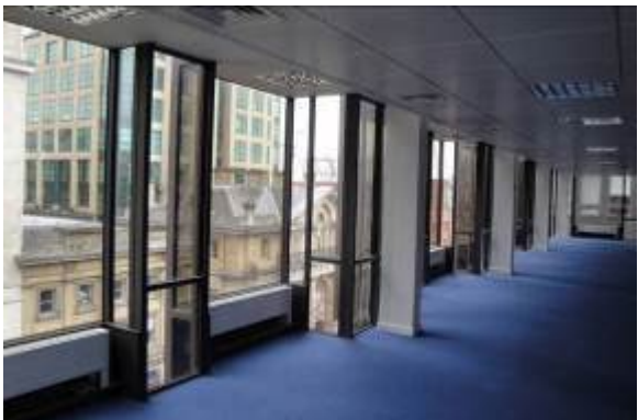
Figure 44: Looking along the King Street Block fenestration, showing the recently lowered suspended ceiling. (Photo taken in 2017; condition has since deteriorated)
