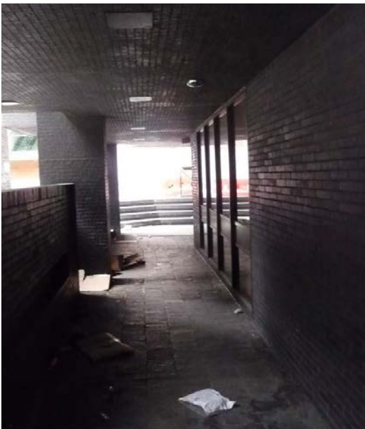
Figure 27b: The appearance and condition of the undercroft former walkway to the eastern side of the piazza as seen in 2022.
