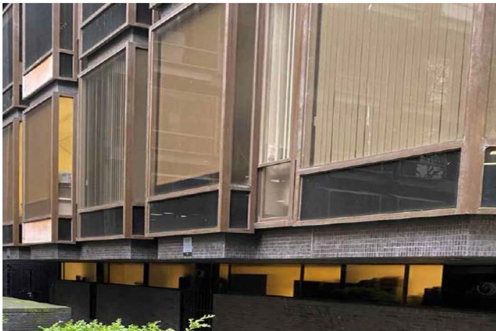
Figure 28: An example of the original windows to the lower parts of the north elevation that looks on to the piazza in 2022, demonstrating the severely deteriorating condition of the 1960s frames, which includes the general poor condition of the now peeling, bubbling and flaking paintwork, subsequent patching and overpainting in gloss paint, failed and broken spandrel panels, deflecting frames and replacement of rubber gaskets with silicon.
