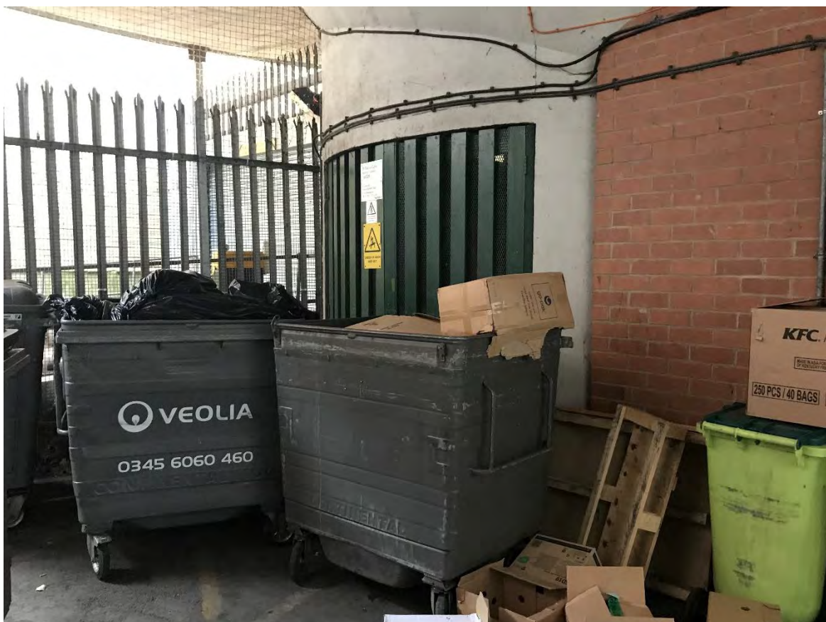
Photo 2: Electric substation to rear of property
