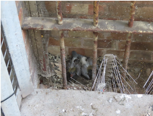
Photograph 4 - Pigeon nest found on floor of car park level during building inspection
