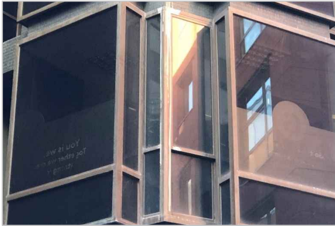
Photograph No. 19 – Excess water staining observed to corner bay (Level 3 – West elevation – Marsden Block)
