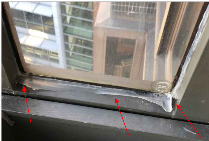
Photograph No. 43 – Clear silicone sealant showing signs of adhesion failure (Level 10 – West elevation – Pall Mall Court)
