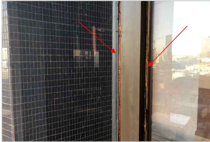
Photograph No. 40 – Sealant degraded between the glazed pane and framework – (Level 10 – West elevation – Pall Mall Court)
