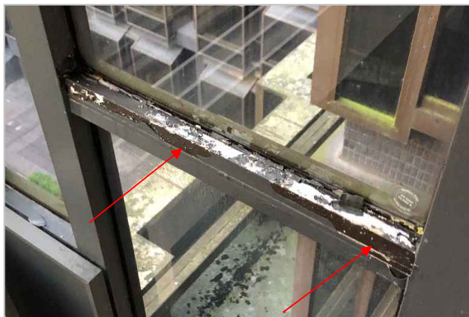
Photograph No. 36 – Degradation to internal paint application exposing bronze PPC (Level 4 – North elevation – King Street Block)
