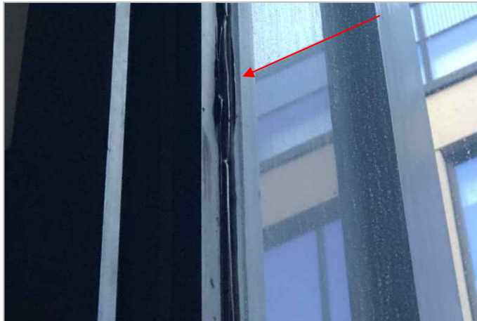
Photograph No. 31 – Deformed seal as a result of age hardening between the glazed pane and framework (Level 2 – South elevation – King Street Block)
