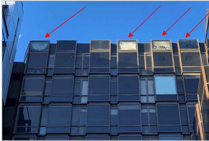
Photograph No. 22 – Spandrel panels at roof level exposed due to degradation of black coating on inside face (Level 10 – East elevation – Pall Mall Court facing Brown Street)
