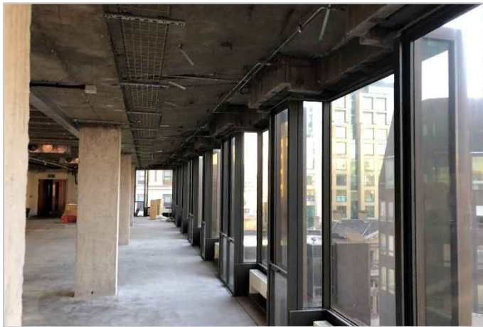
Photograph No. 7 – Underside of slab exposed revealing the installation methodology of aluminium shopfront system
