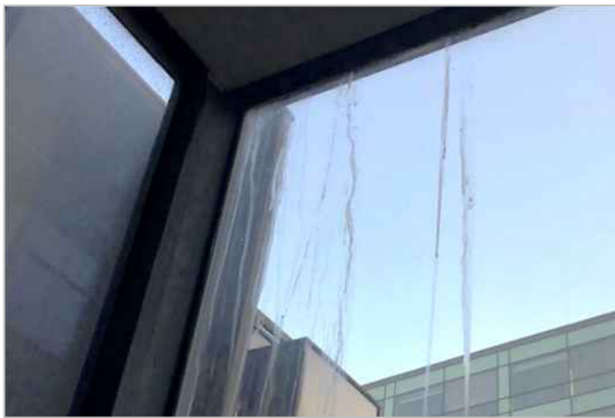
Photograph No. 47 – A number of water streaks on glazed pane (Level 2 – West elevation – Pall Mall Court)
