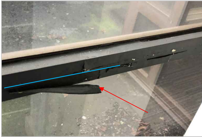
Photograph No. 35 – Paint peeling away from framework (Level 3 – South elevation – King Street Block)
