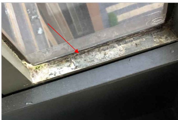
Photograph No. 39 – Heavy degradation to framework (Level 9 – West elevation – Pall Mall Court)
