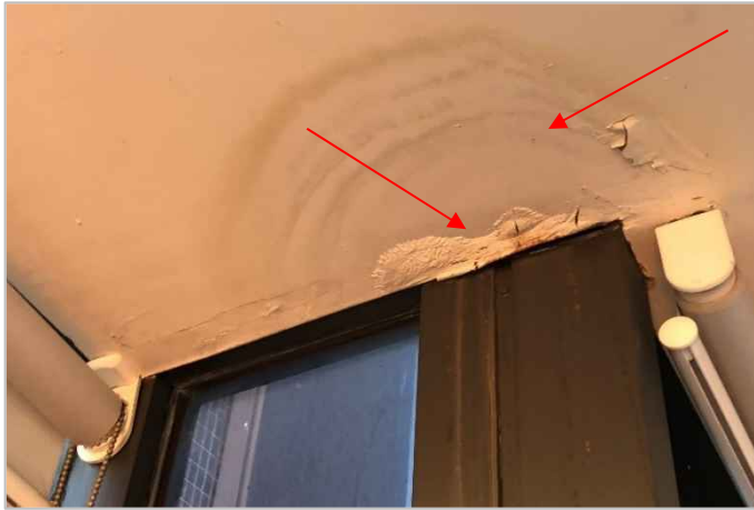
Photograph No. 52 – Excessive water damage to ceiling (Level 10 – East elevation – Pall Mall Court)
