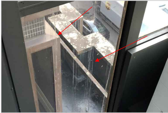
Photograph No. 48 – Water streaks observed to glazed pane (Level 4 – South elevation – King Street Block)
