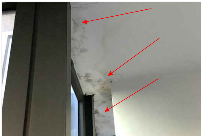
Photograph No. 51 – Water staining to ceiling (Level 4 – West elevation – Marsden Block)
