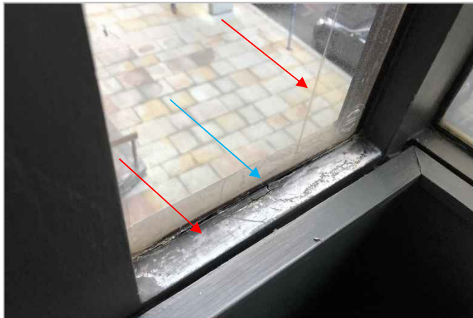
Photograph No. 32 – Degradation of paint and sealant applied (Level 1 – South elevation – King Street Block)
