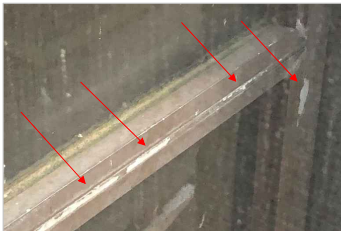
Photograph No. 16 – Paintwork applied to framework observed peeling from edges on framework (Level 3 – East elevation – Pall Mall Court)
