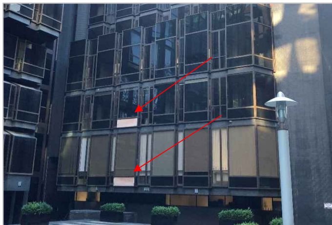
Photograph No. 25 – Glazed spandrel panels replaced with timber boards (Levels 1 & 2 – North elevation – King Street Block)
