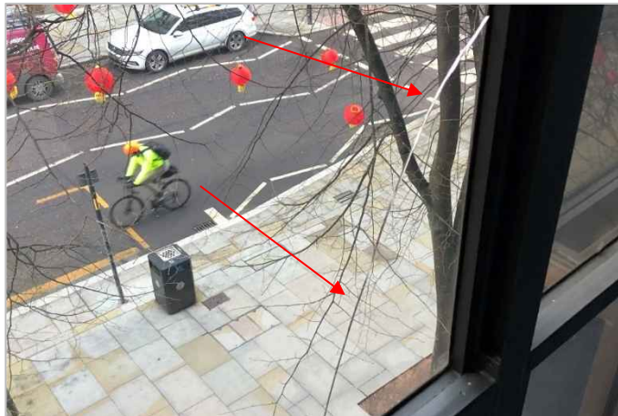
Photograph No. 30 – Internal view of cracked glazed pane (Level 1 – South elevation – King Street Block)
