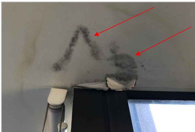
Photograph No. 53 – Black mould observed to ceiling around glazing system (Level 10 – West elevation – Pall Mall Court)
