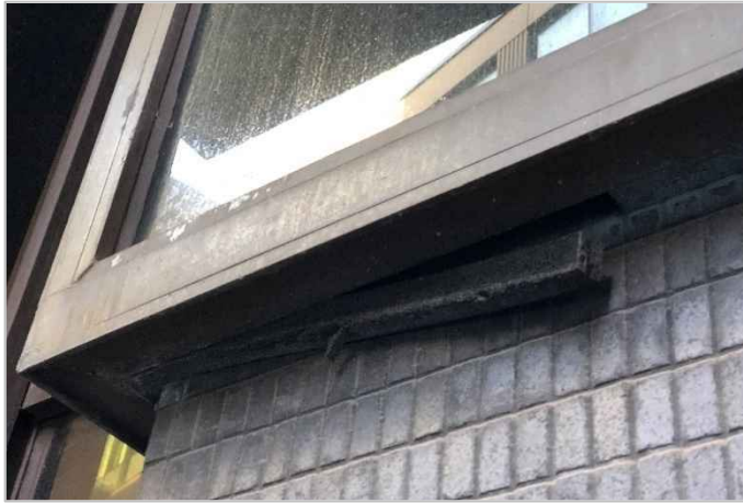
Photograph No. 29 – Impregnated foam found loose between façade and glazing system (Level 1 – West elevation – Marsden Block)
