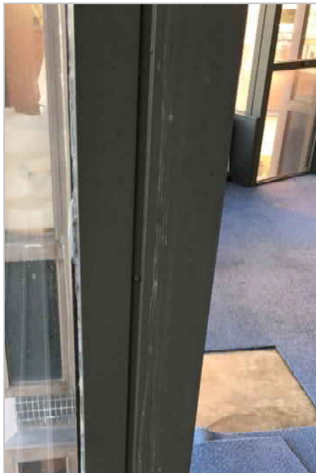
Photograph No. 49 – Water staining found on the framework (Level 10 – North elevation – Pall Mall Court)
