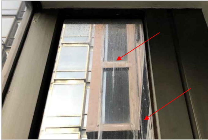
Photograph No. 46 – Water streaks on glazed pane (Level 2 – North elevation – Marsden Block)
