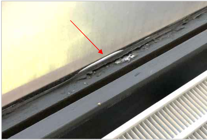
Photograph No. 41 – Adhesion failure of sealant applied to framework and glazed pane (Level 10 – East elevation – Pall Mall Court)
