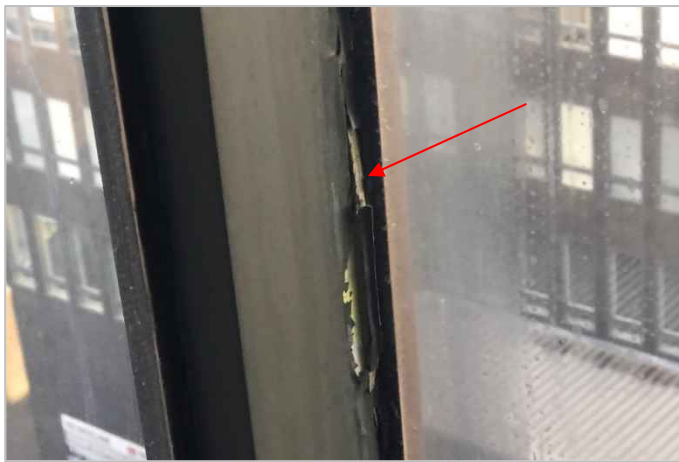
Photograph No. 38 – Sealant applied degraded with paint work flaking (Level 9 – West elevation – Pall Mall Court)
