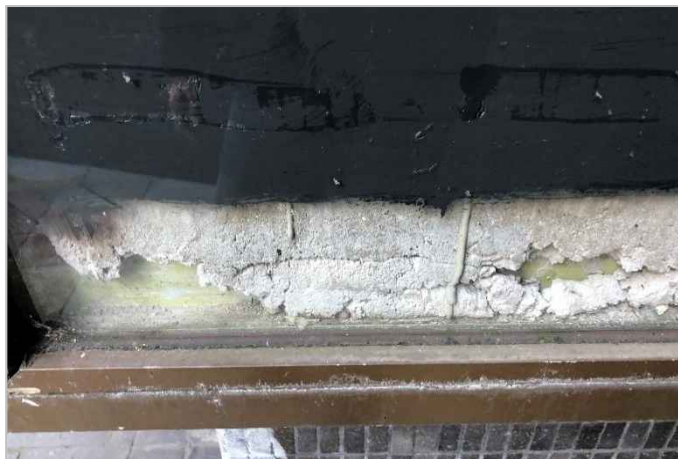
Photograph No. 21 – Black coating to spandrel panel degraded, exposed materials behind it (Ground floor – South elevation – King Street)
