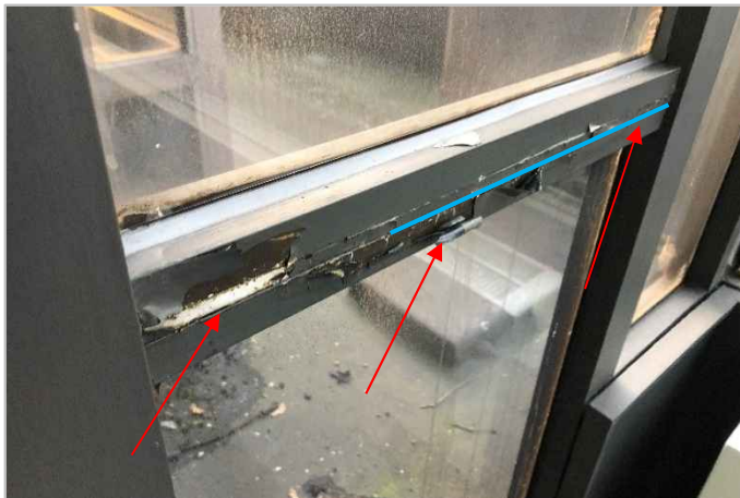
Photograph No. 34 – Paint application peeling away from the framework (Level 3 – South elevation – King Street Block)
