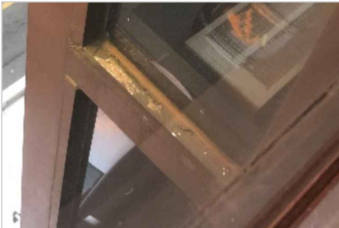
Photograph No. 18 – Water damage to framework (Level 2 – North elevation – Marsden Block)
