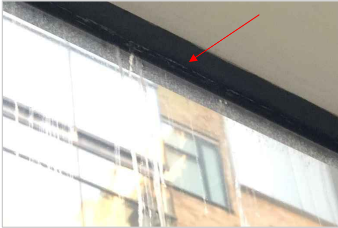
Photograph No. 44 – Water streak from under glazing seal (Level 2 – North elevation – Marsden Block)
