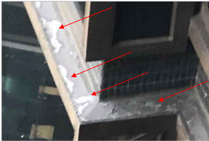
Photograph No. 15 – Paintwork deteriorated on top of framework (Level 6 – West elevation – Pall Mall Court)
