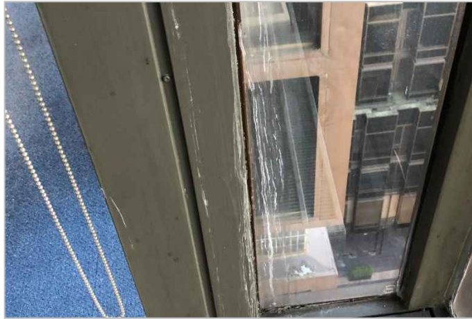
Photograph No. 50 – Heavy water staining to framework and glazed pane (Level 10 – West elevation – Pall Mall Court)
