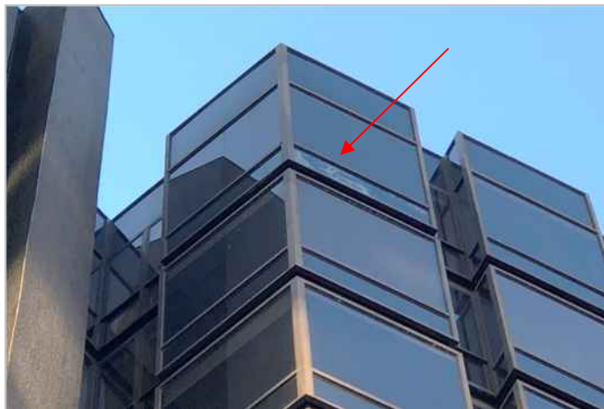
Photograph No. 23 – Black coating to spandrel panel deteriorated over time (Level 5 – North elevation – Marsden Block)
