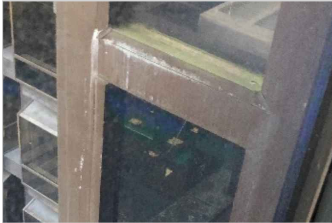
Photograph No. 17 – Water staining observed to framework (Level 4 – South elevation – Marsden Block)
