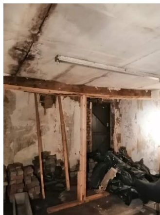
Photograph 9: Observed damp in basement
