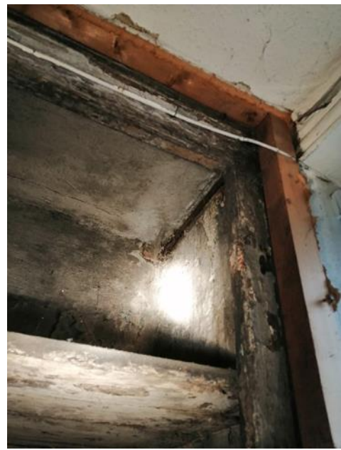
Photograph 5: Southern aspect of B1 with exposed gaps leading to the floor above
