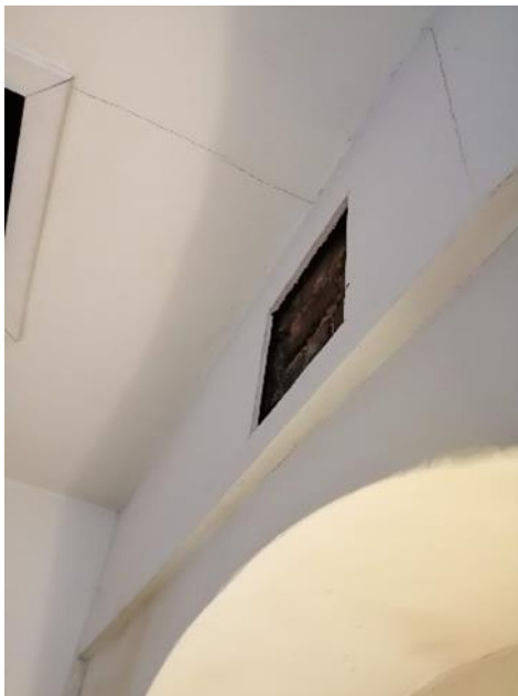
Photograph 6: Exposed plasterboard crevice adjacent to loft access
