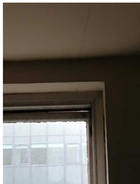
Photograph 7: Top floor gap in window pane
