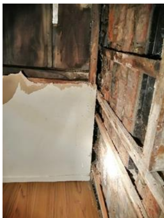
Photograph 12: Exposed brickwork and plasterboard with damp observed
