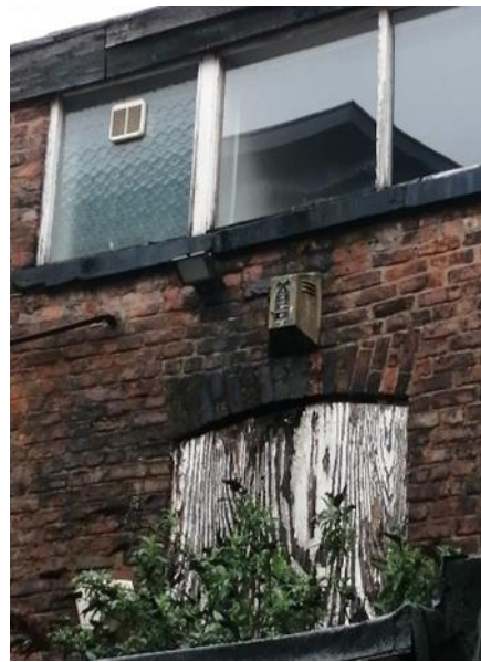
Photograph 2: Southern aspect of B1 with exposed gaps
