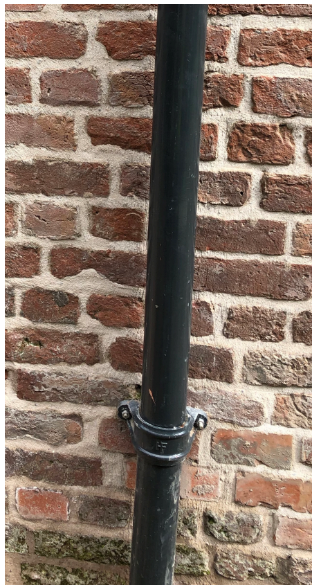
replacement cast iron pipework as installed for site inspection
