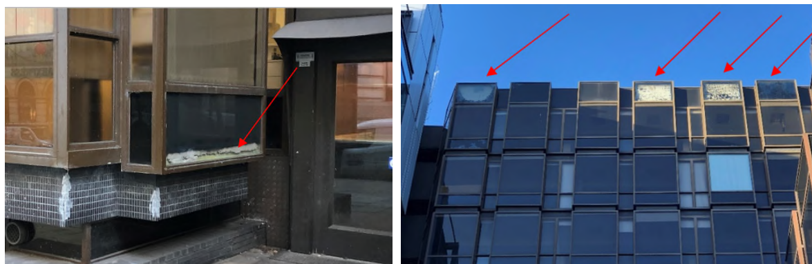
Figure 4.3: Examples of Failed Curtain Walling
