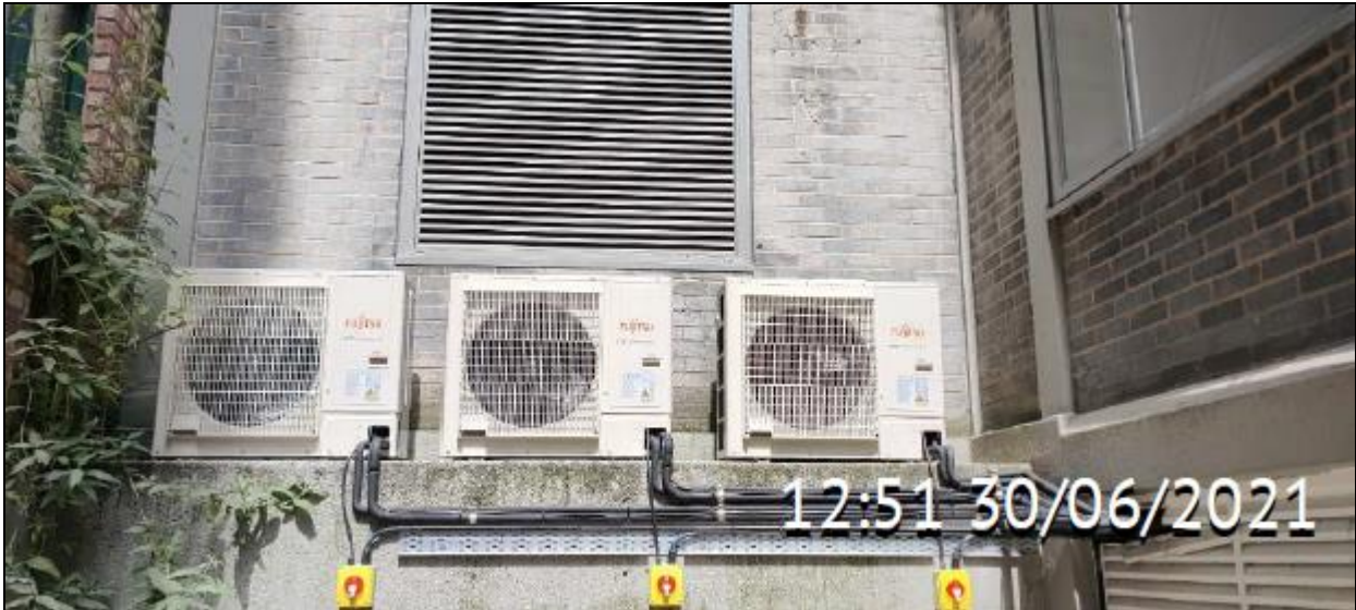
Figure 2: Photograph of three external air conditioning units.
