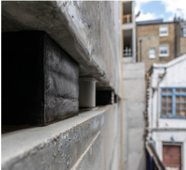
Figure 5 – Isolation bearings and bespoke lateral restraint system
