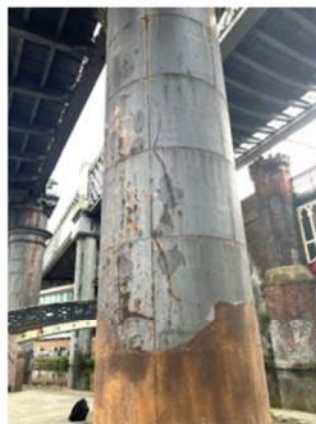
Figure 10 – Location 1 - example of main pier crack
