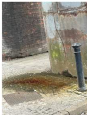
Figure 9 - Example of constant drip patch under downpipe joint.
