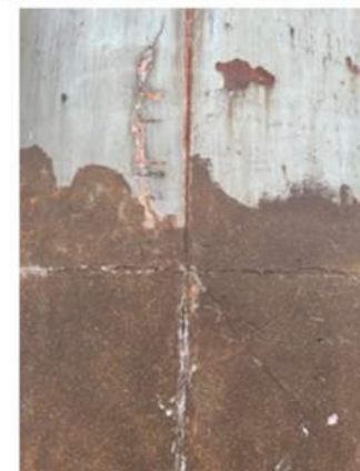
Figure 11 - Location 2 - example of main pier crack
