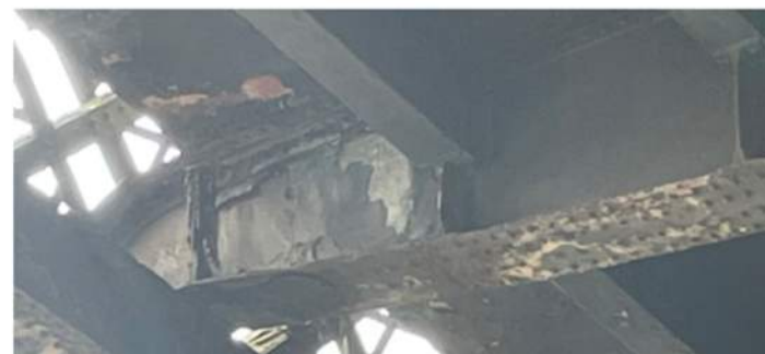
Figure 4 - Example of significant corrosion and possible delamination of the end web stiffener on the fish-belly beams
