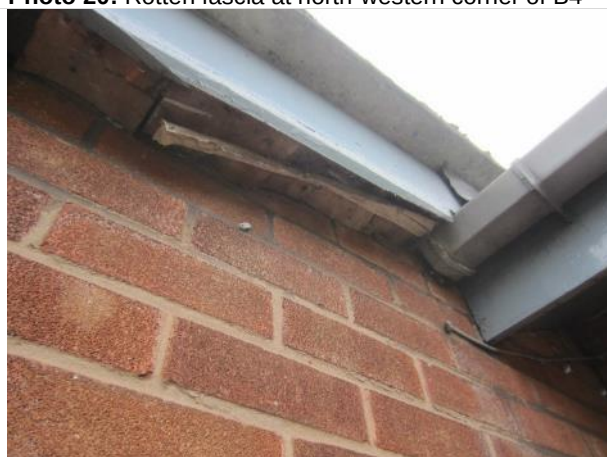
Photo 22: Rotten timber at eaves of B4
