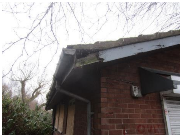
Photo 20: Rotten fascia at north-western corner of B4
