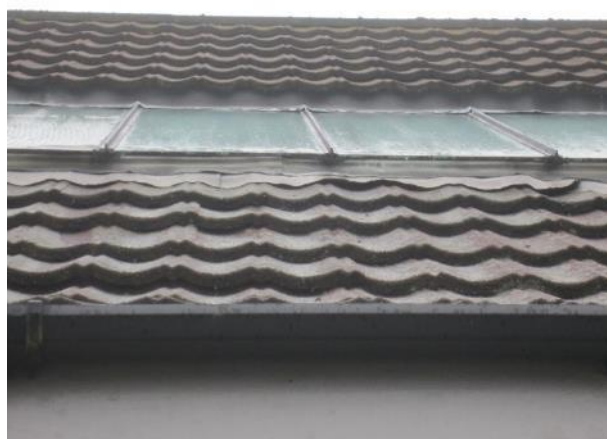
Photo 30: Skylights and lifted flashing at B7
