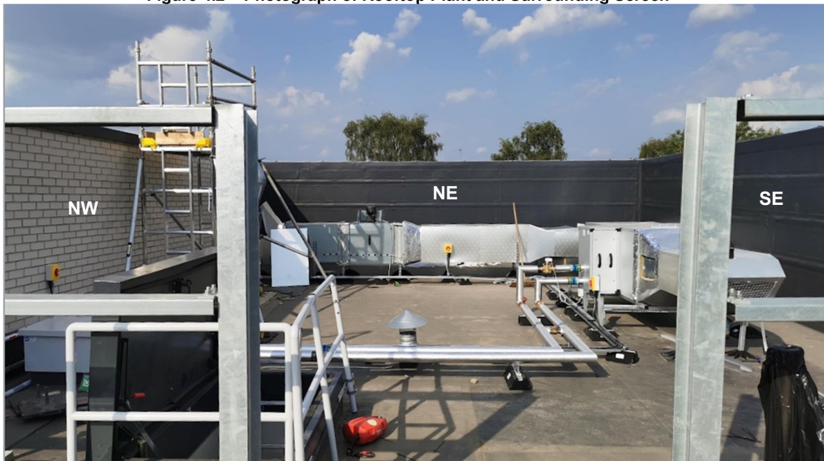
Figure 4.2 – Photograph of Rooftop Plant and Surrounding Screen
