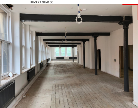
PHOTOGRAPH OF GENERAL AREA SHOWING HOW THE EXISTING FLOOR JOISTS ABOVE HAVE BEEN UNDERDRAWN WITH MODERN PLASTERBOARD AND SKIM FINISH, PAINTED WITH WHITE EMULSION AND THE SUBSEQUENT INSTALLATION OF MODERN SPOT DOWNLIGHTERS (WHICH ARE INAPPROPRIATE FOR OFFICE USE) MAIN SUPPORT BEAMS LEFT EXPOSED WITH PAINT FINISH.
