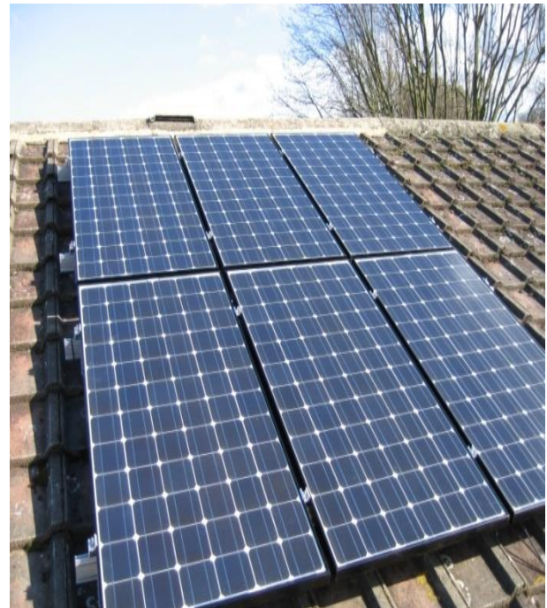
Figure 5 - Photovoltaic array on a pitched roof
