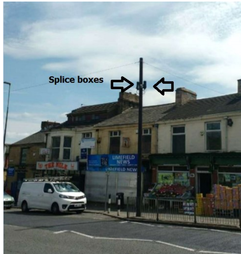
Figure 2: Photograph of splice boxes commonly seen on poles supporting fibre
