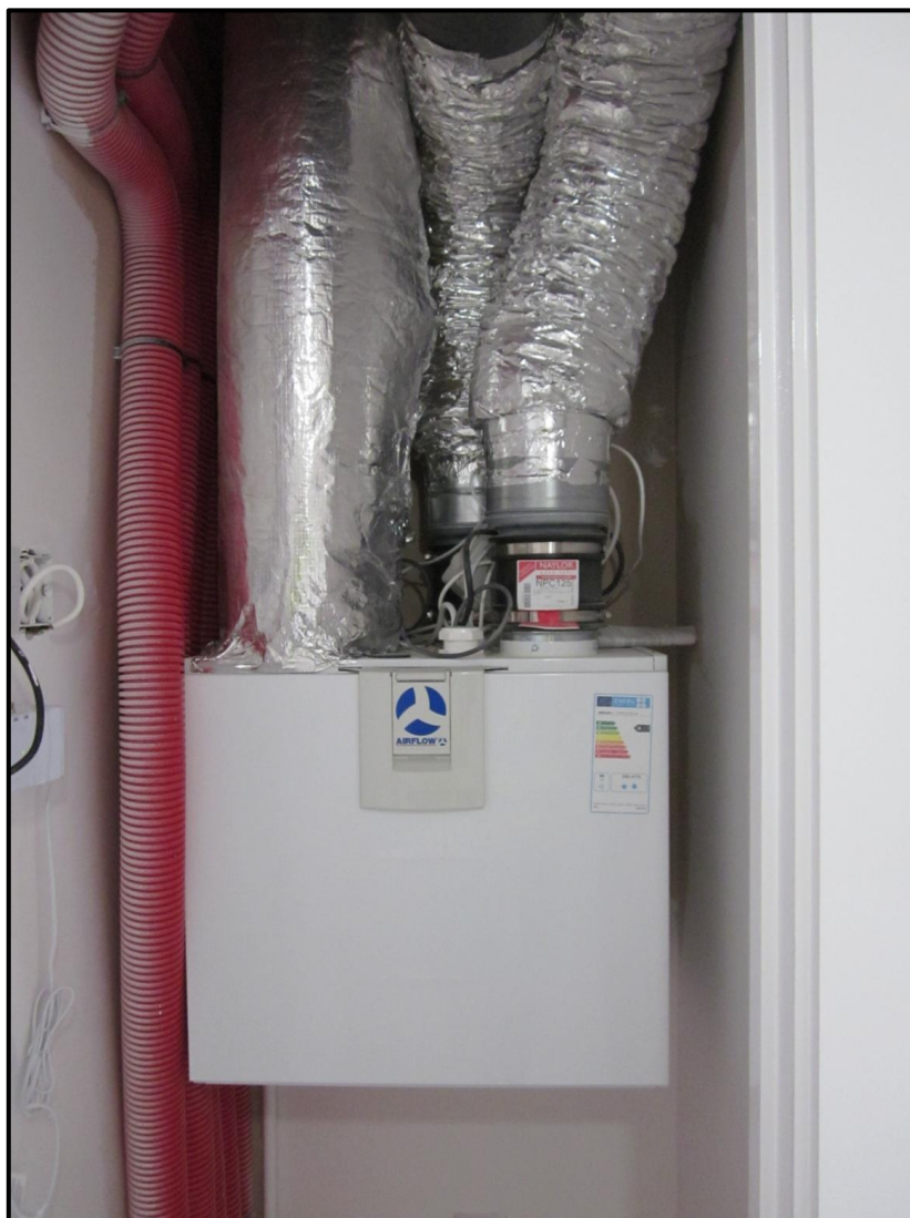
Photograph 4. MVHR system used throughout the development
