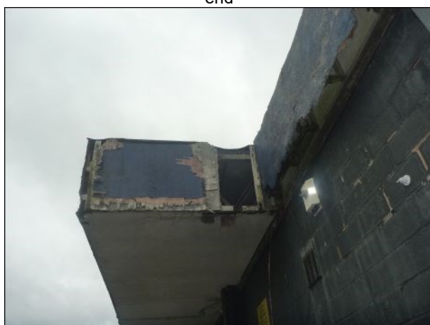
Photo 9: Building 1, damage to timber canopy roof
