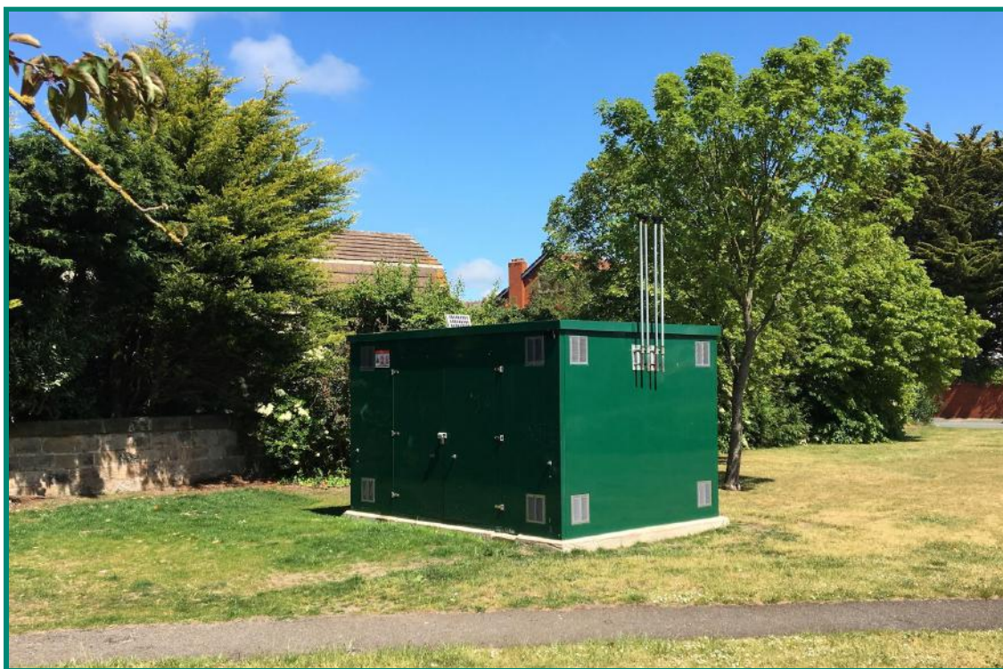
Figure 2 - Example of a similar gas governor and kiosk
