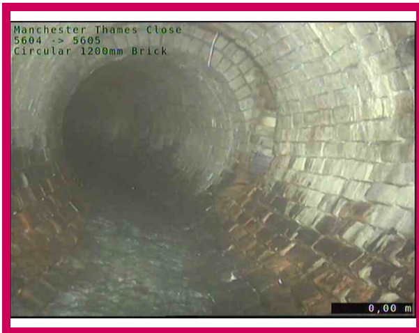
1, 00:00:04, 0.00 m Mortar missing, from 15 to 50 mm mortar loss from 04 o'clock to 07 o'clock, start
