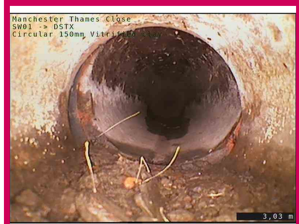
2, 00:01:08, 3.03 m Joint displaced, medium
