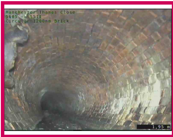
1, 00:00:16, 1.95 m Connection defective, connecting pipe is intruding at 10 o'clock, diameter: 675mm, intrusion: 10%
