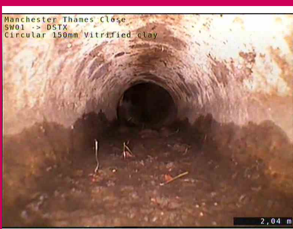
1, 00:00:23, 1.78 m Settled deposits, fine, 10% cross-sectional area loss
