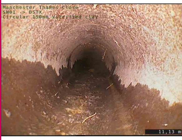
3, 00:03:56, 11.13 m Settled deposits, fine, 10% cross-sectional area loss
