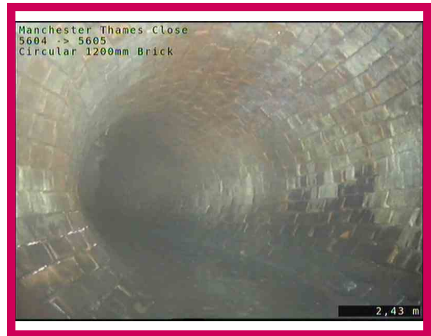
2, 00:00:31, 2.43 m Mortar missing, from 15 to 50 mm mortar loss from 4 o'clock to 7 o'clock, finish
