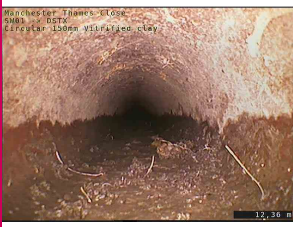
5, 00:04:11, 12.36 m Survey abandoned, Debris silt 15%
