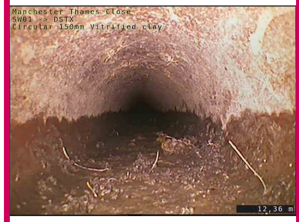
4, 00:04:03, 11.94 m Settled deposits, fine, 15% cross-sectional area loss
