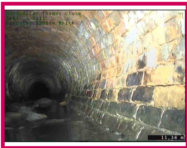
3, 00:02:11, 9.95 m Settled deposits, coarse, 15% cross-sectional area loss
