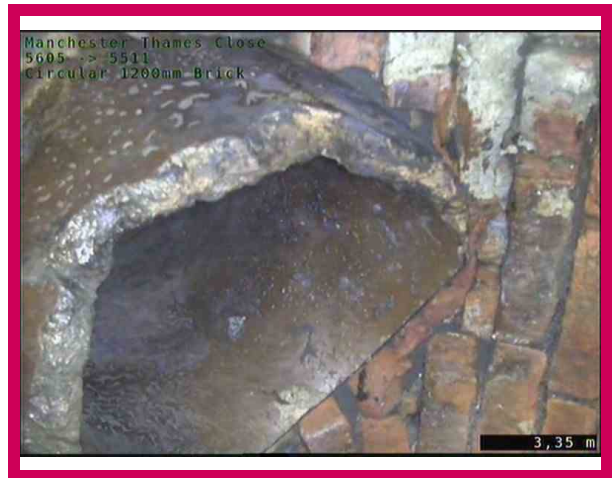
2, 00:00:29, 3.35 m Connection defective, connecting pipe is intruding at 9 o'clock, diameter: 300mm, intrusion: 10%
