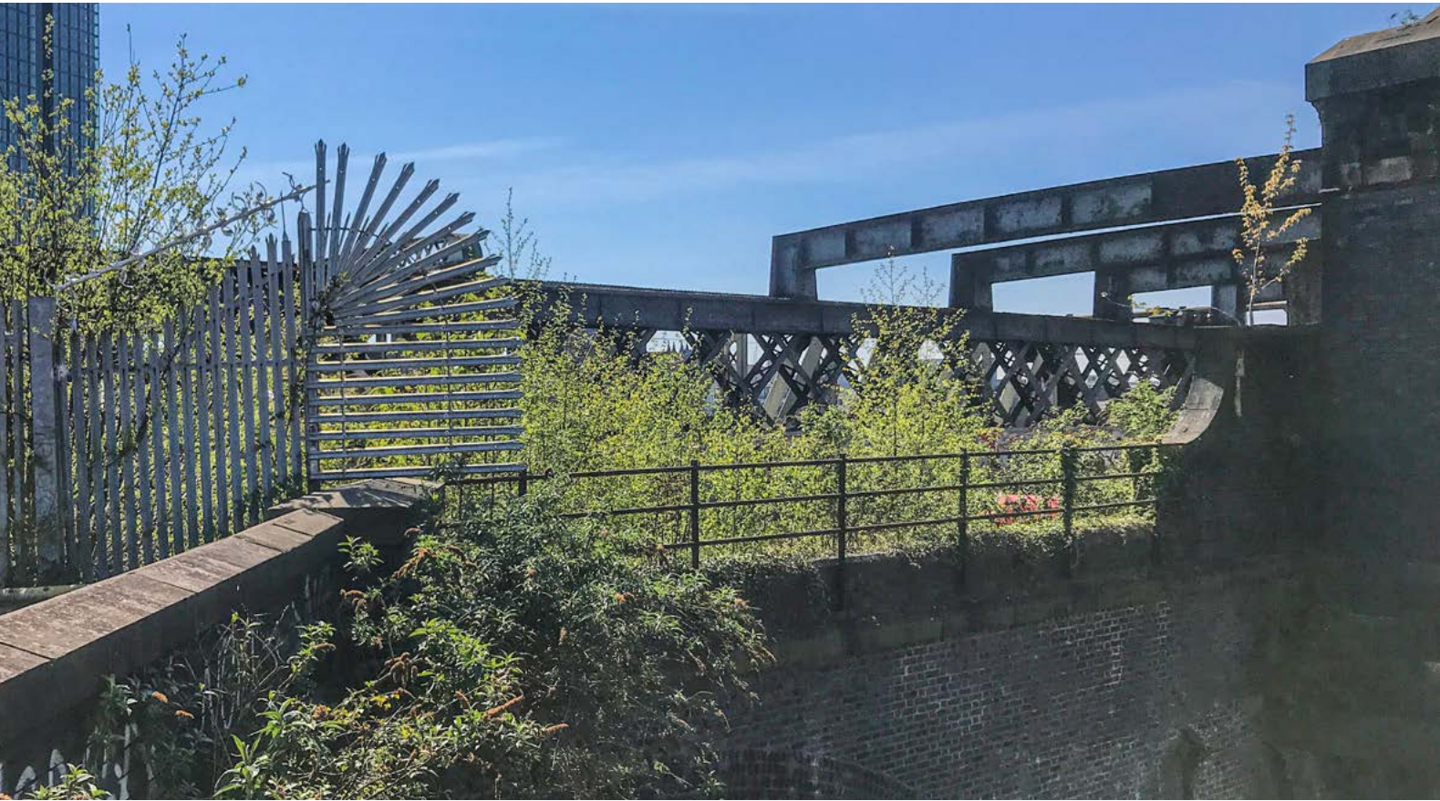
Photo of existing, inadequate guarding
