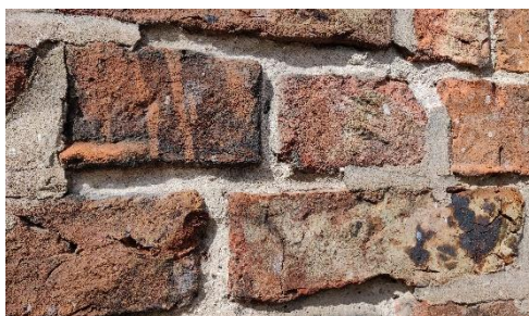
Area of brickwork showing where the cement mortar has failed, and the underlying lime mortar is visible
