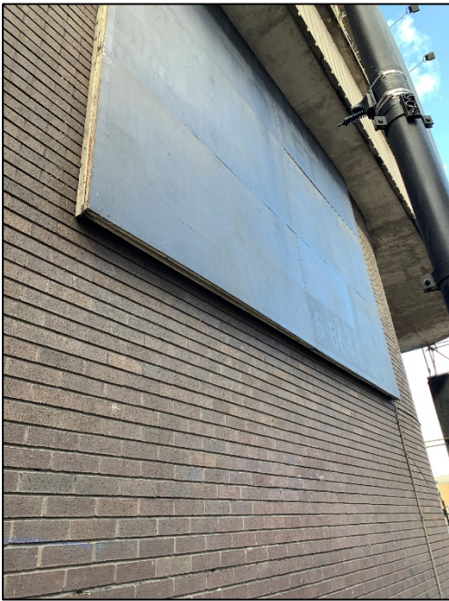
Photo 9 Wooden boarding on east face
