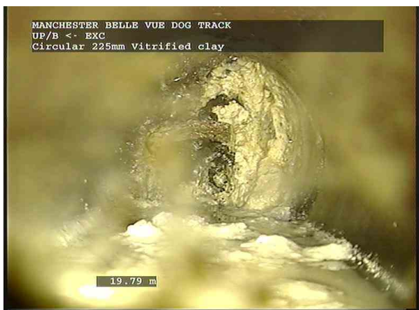
UP_BX_6a5f76b5-5bea-4fbb-9ef3-7b1d99de9668_20211115_103042_596.jpg, 00:05:45, 19.79 m Survey abandoned, COLLAPSED
