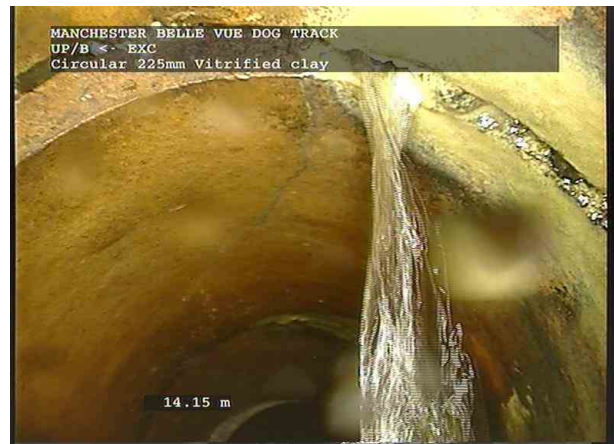
UP_BX_f80be6bf-109d-46c3-9c52-611f2be35c0d_20211115_102636_062.jpg, 00:02:54, 14.15 m Infiltration, running at joint at 1 o'clock
