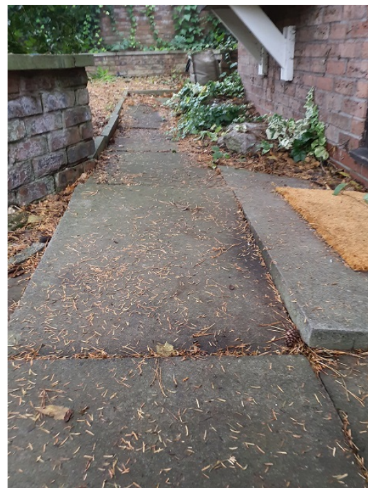
Figure 3. Paving appears to be affected by roots
