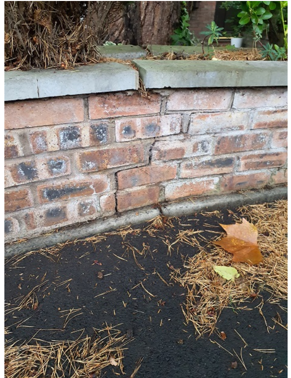
Figure 4. Crack forming in front wall
