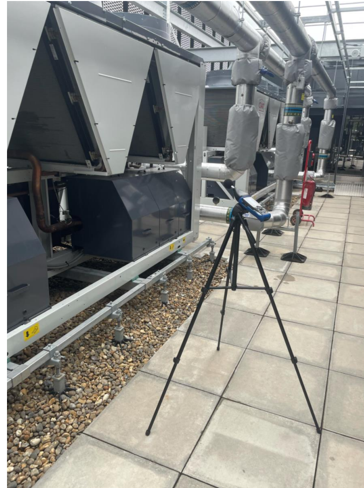
Photograph of SLM for source level measurement adjacent to Chiller 1
