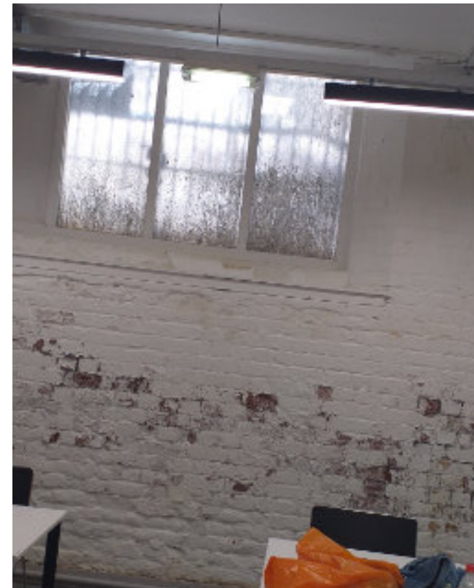
Existing damp issues within the basement
