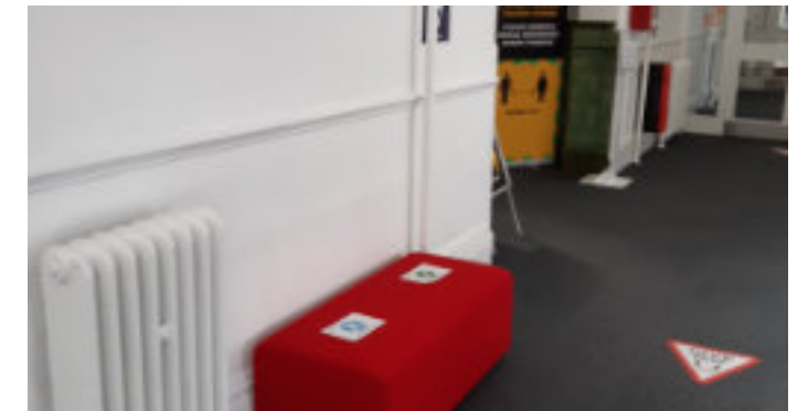
Ground Floor Circulation - Radiators
