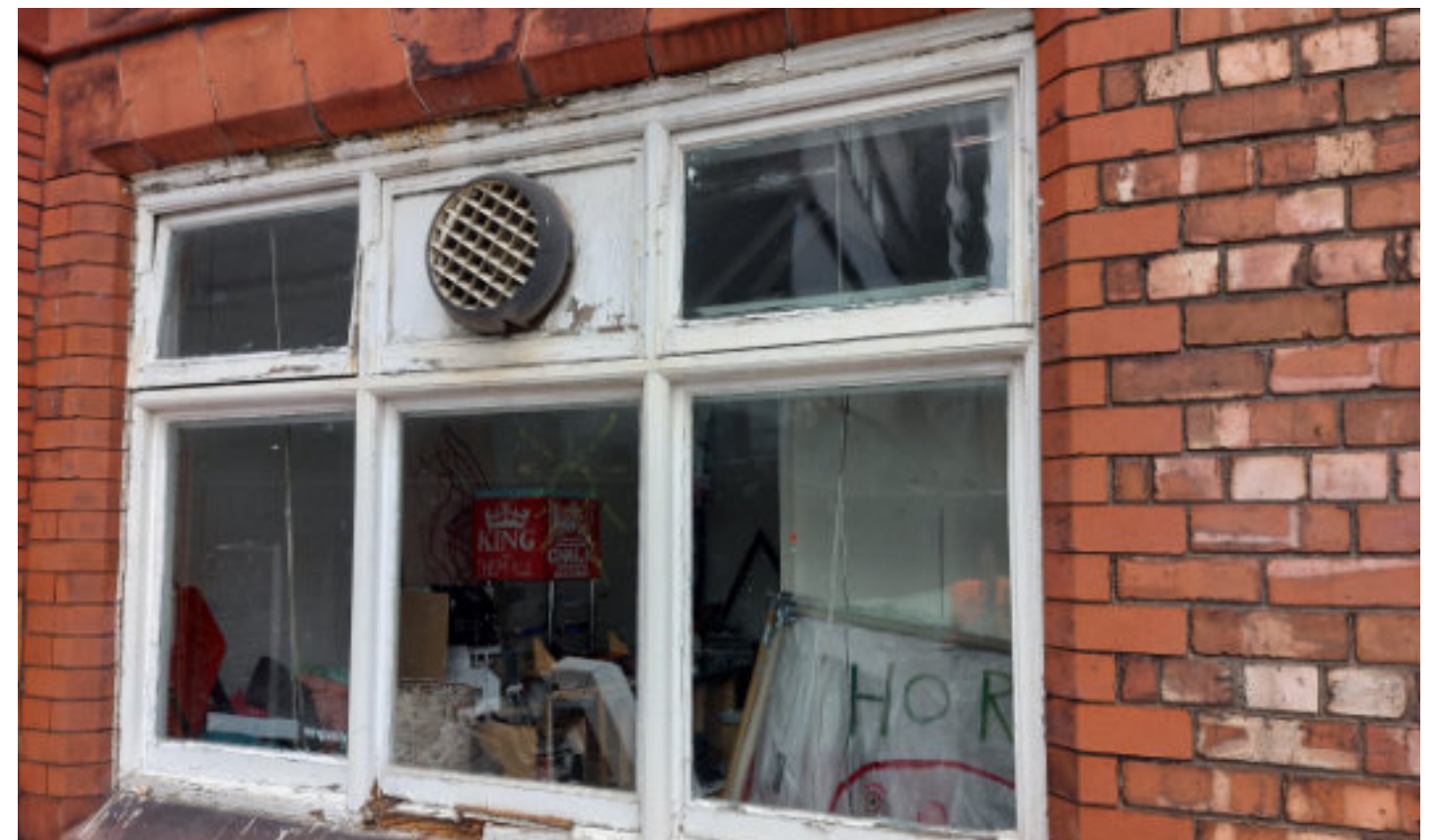
Example of timber rot & decay to window frames for resin repair of rail replacement (cill) - modern services infill
