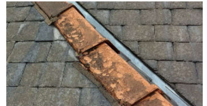
Ridge tile surface degrading
