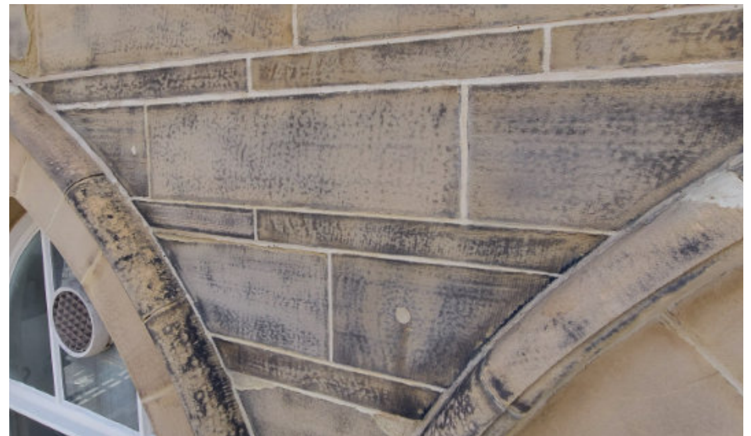
Higher Ormond Street Elevation - Failing mortar to be restored
