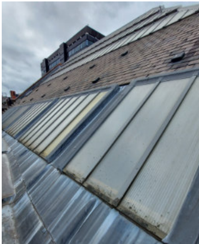
Degrading aluminium rooflight & polycarbonate light
