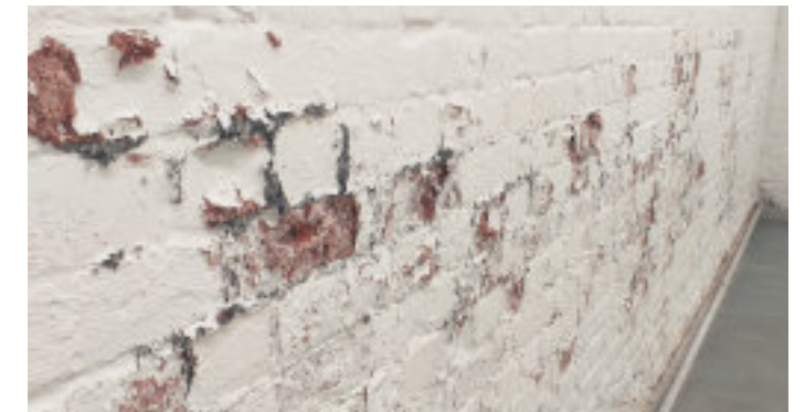
Existing damp issues within the basement
