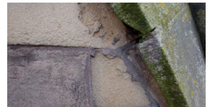
Incorrect hard cementitious mortar
