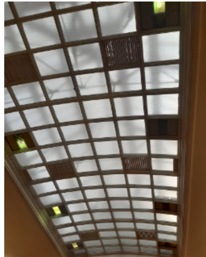
Holden Gallery - Lay-In Lights with services
