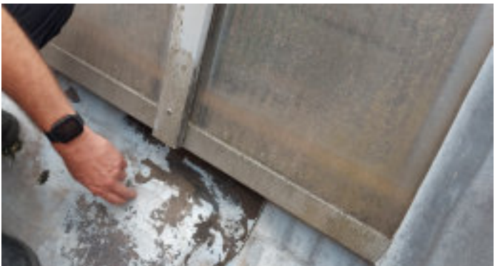
Mastic split repairs to lead
