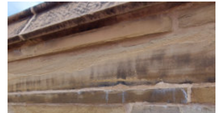
Salting or calcium deposits on parapet pointing
