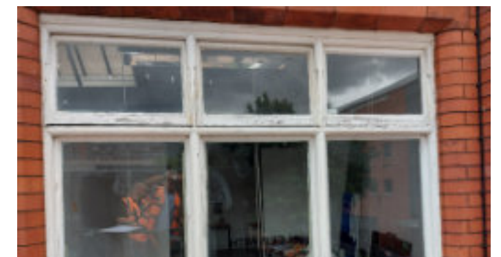
Flaking paint and missing beading
