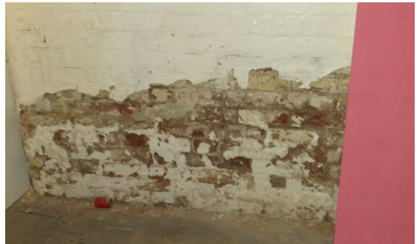
Existing damp issues within the basement
