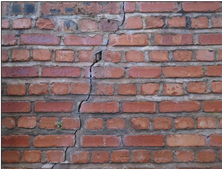
Photograph 6 showing the crack in the wall
