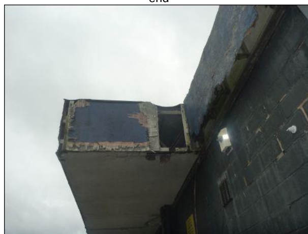
Photo 10: Building 1, damage to timber canopy roof
